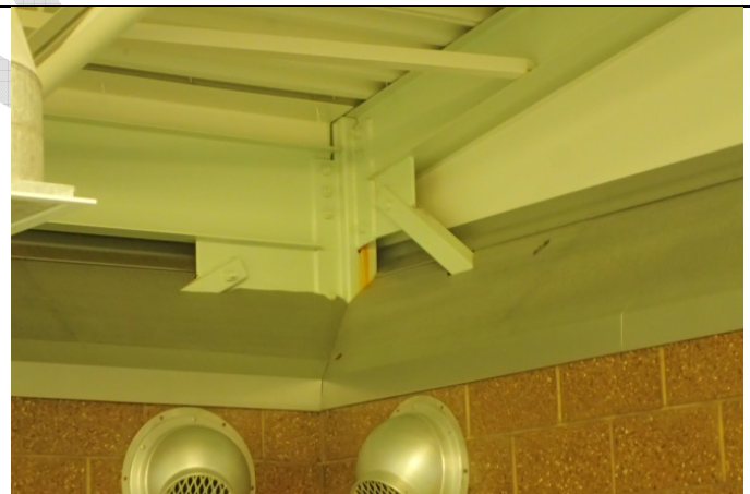
Figures -3.1b Rust noted on Column A:1.
