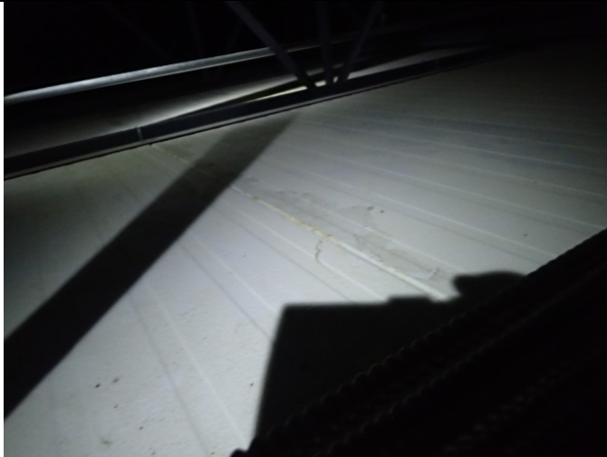
Fig. 1.2a. Likely missing butyl tape at panel joint. Note frost on either side of joint.
