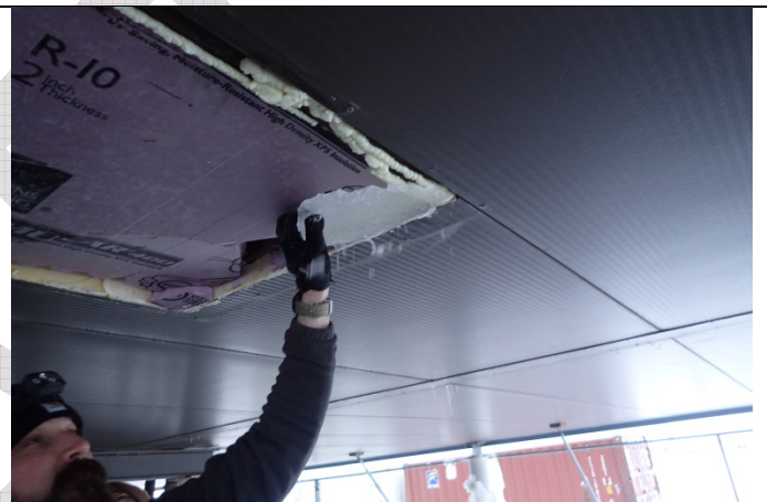
Fig. 1.4b. Ice present at access door cut into soffit panel.
