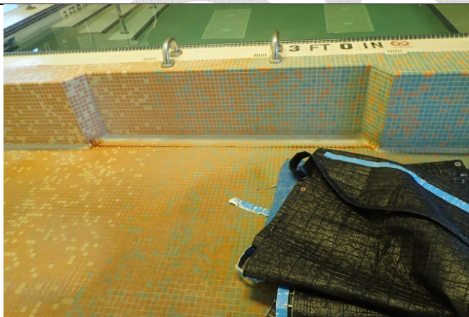
Fig. 5a. Pool cover results in standing water, staining of tile and grout, and saturation of concrete deck to rebar below.
