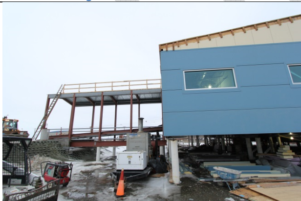
Fig. 2.1d. Rake condition above Conference Room 102, as seen on April 3, 2014 Construction Observation Site Visit.
