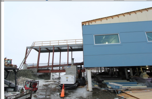
Fig. 2.1d. Rake condition above Conference Room 102, as seen on April 3, 2014 Construction Observation Site Visit.
