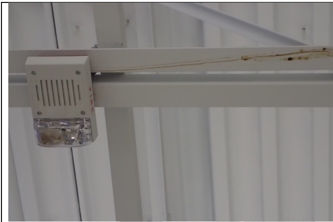
Fig. 3.2a. Damaged strobe/annunciator. Inspect to ensure it is still operational and replace if not. Install metal flashing to divert leaking from causing further damage.
