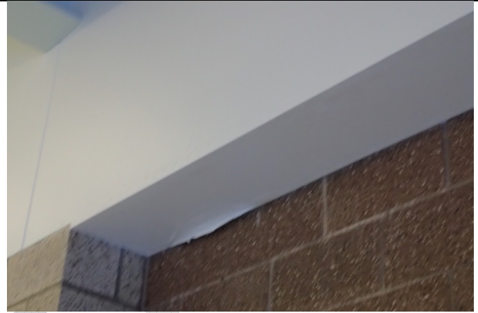
Fig. 3.1d. Damaged GWB at bulkhead near Grid G:2.
