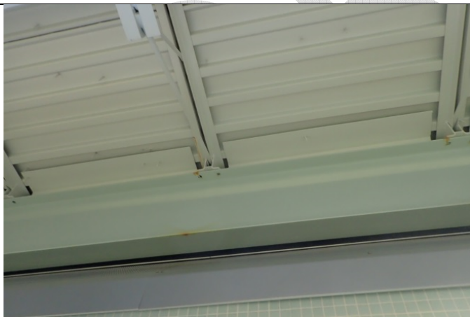
Fig.3.1a. Small areas of rust on open web joists and wide flange, associated with leaking roof.
