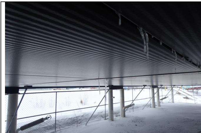
Fig. 1.4a. Significant amounts of ice at panel joints where water had leaked from burst piping.
