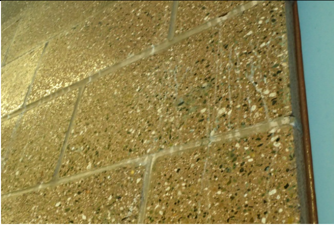
Fig. 3.1c. Efflorescence on CMU and Grout near Pool Equipment Storage
