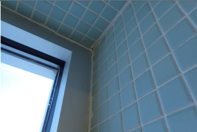
Fig. 3.1e. Cracked tile in soffit of window well. Cracks may be associated with water damage, but may also be associated with building movement. Monitor for further movement.
