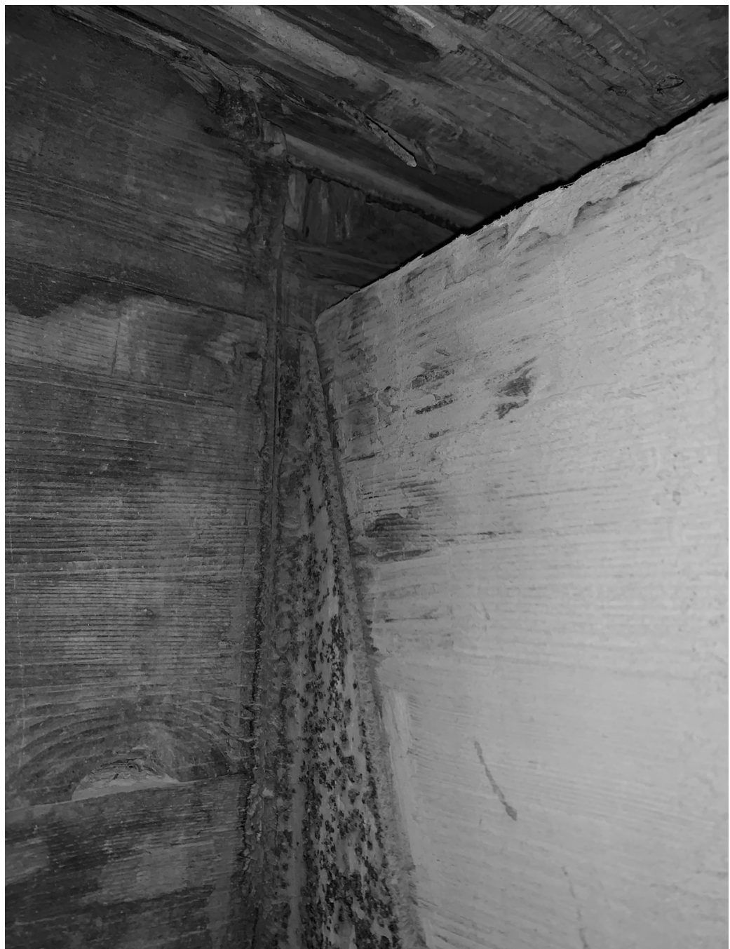
FAILED BEAM HANGER NOT TO SCALE
