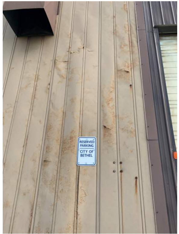
Photo 6 – Corroded Wall Panel
