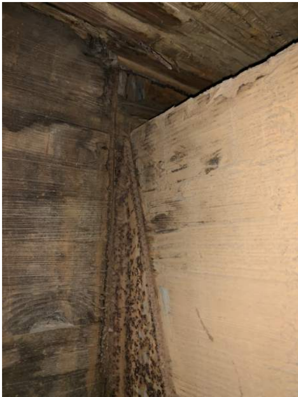
Photo 3 – Failed Beam Hanger
