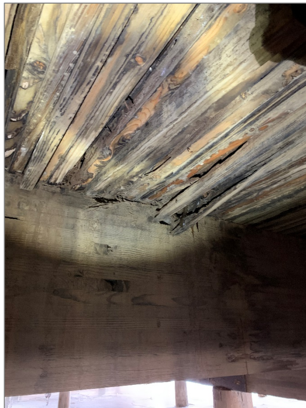
Figure: 12 – Rotting subfloor
