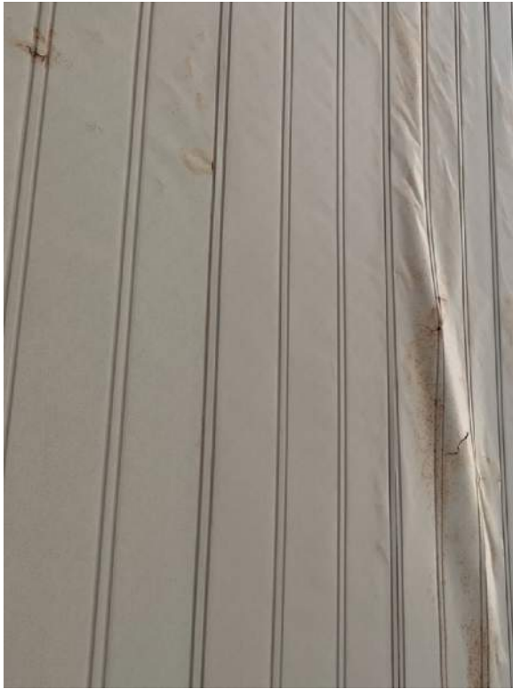
Photo 5 – Failed Wall Panel
