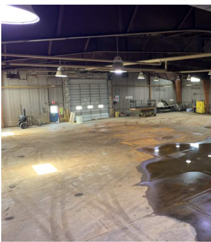
Photo 1 – Standing water on floor deck
