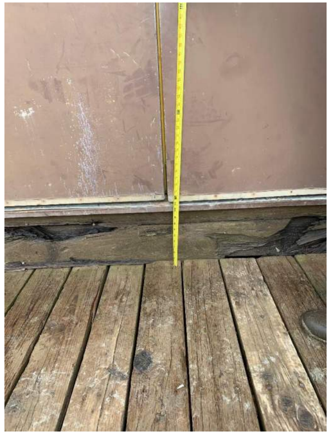
Photo 10 – Step Height at Building Entrance (11")
