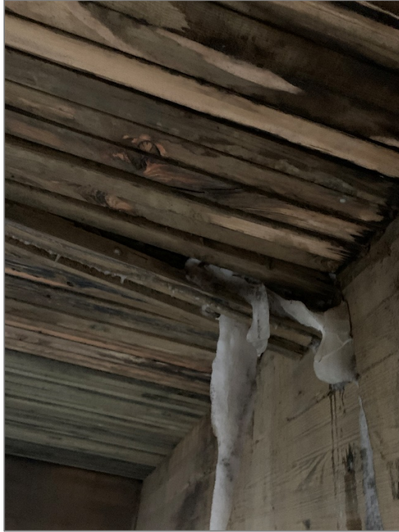
Figure: 13 – Rotting subfloor
