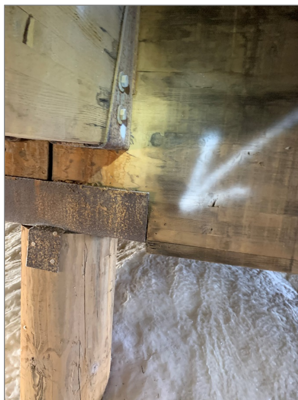
Figure: 8 – Wood piling and twisted floor joist
