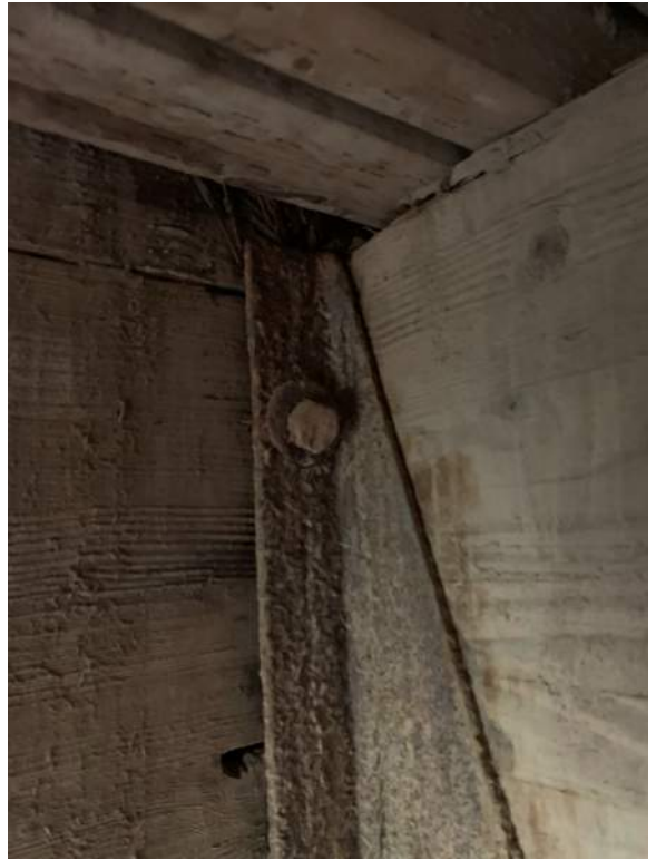
Photo 2 – Failed Beam Hanger
