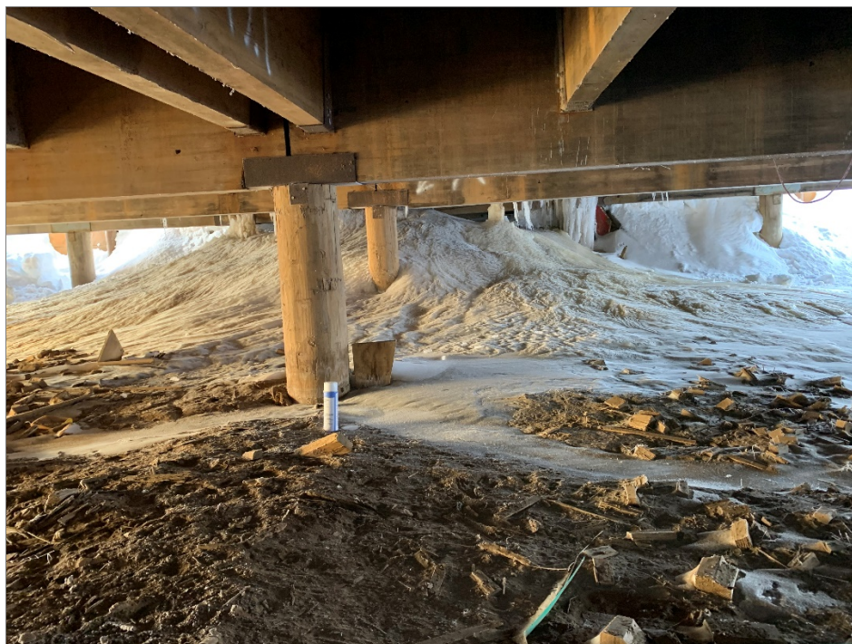
Figure: 7 – Result from leaking floor
