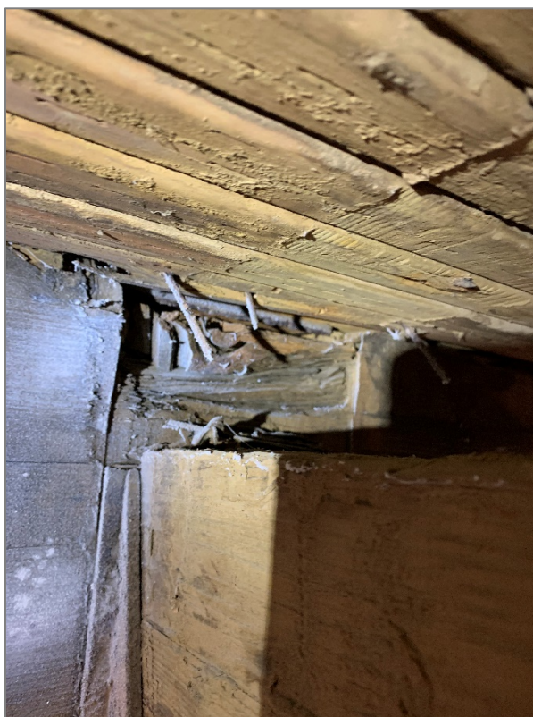
Figure: 10 – Subfloor and rotting floor joist
