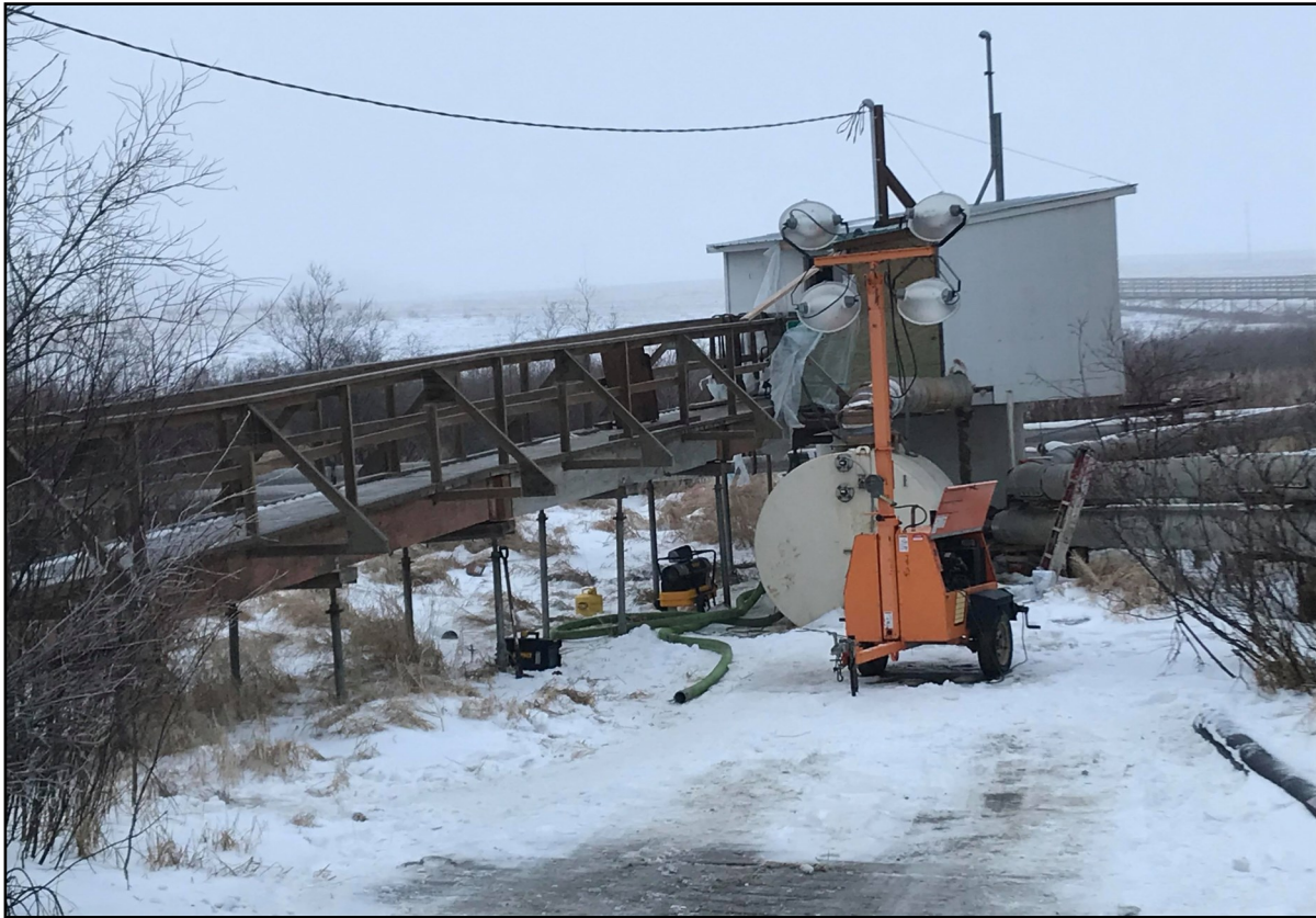
Walking ramp leads to Bethel Main Lift Station that serves Bethel Heights Subdivision. Green hoses and equipment on the ground. Orange light bank allows work to be done in early morning and evening.
