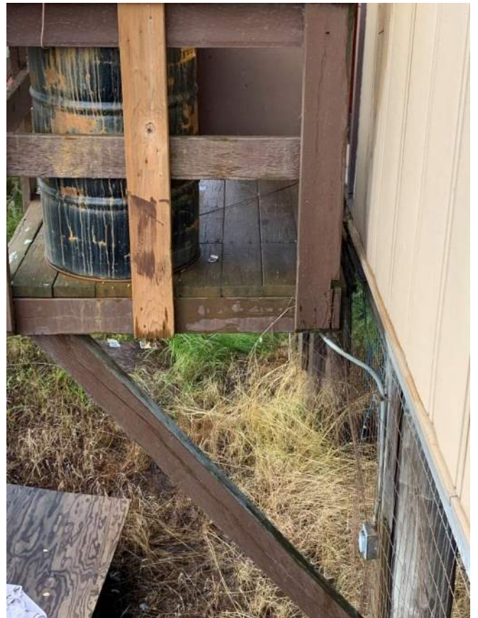
Photo 8 – Exterior Deck – Unsafe
