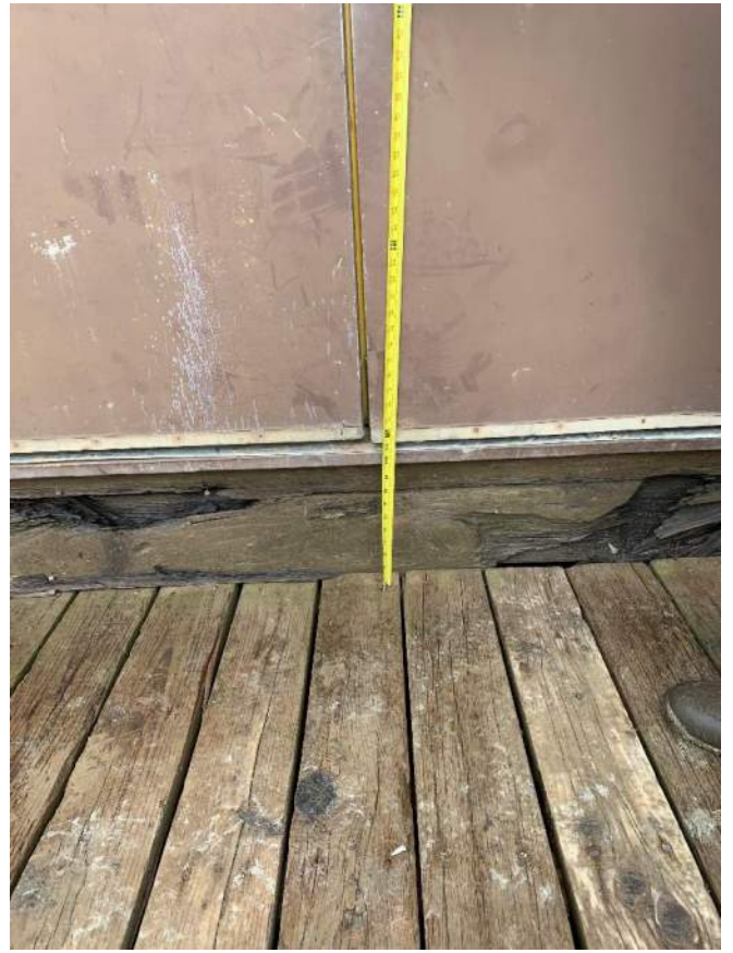
Photo 10 – Step Height at Building Entrance (11")
