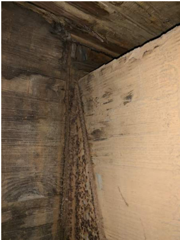
Photo 3 – Failed Beam Hanger
