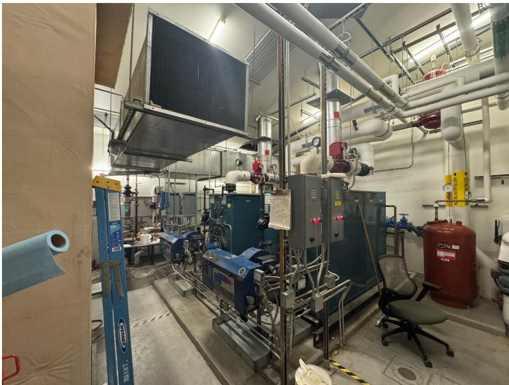
Boiler room, well insulated piping
