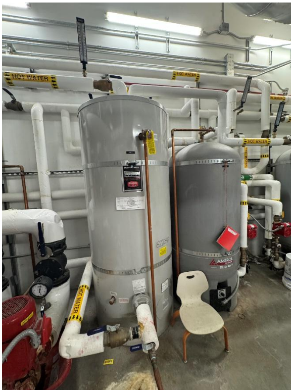
Indirect hot water generator and storage tank
