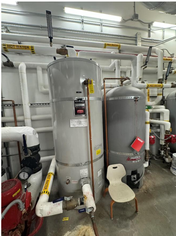
Indirect hot water generator and storage tank
