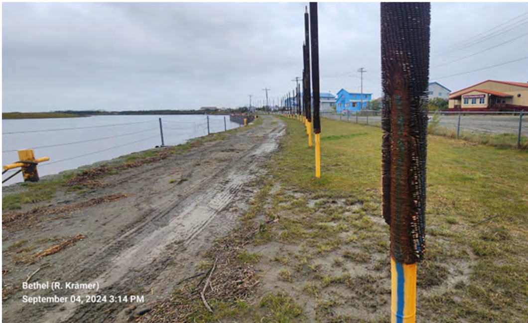
Photo 16: Rusted condition of cooling fins on thermotubes (also known as thermosiphons), Approx. PBL STA 77+00
