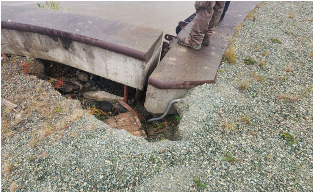
Photo 26: Alternate view of failed area of piles adjacent to City Dock, photo taken 4 September 2024 at 1543, Approx. PBL STA 93+40
