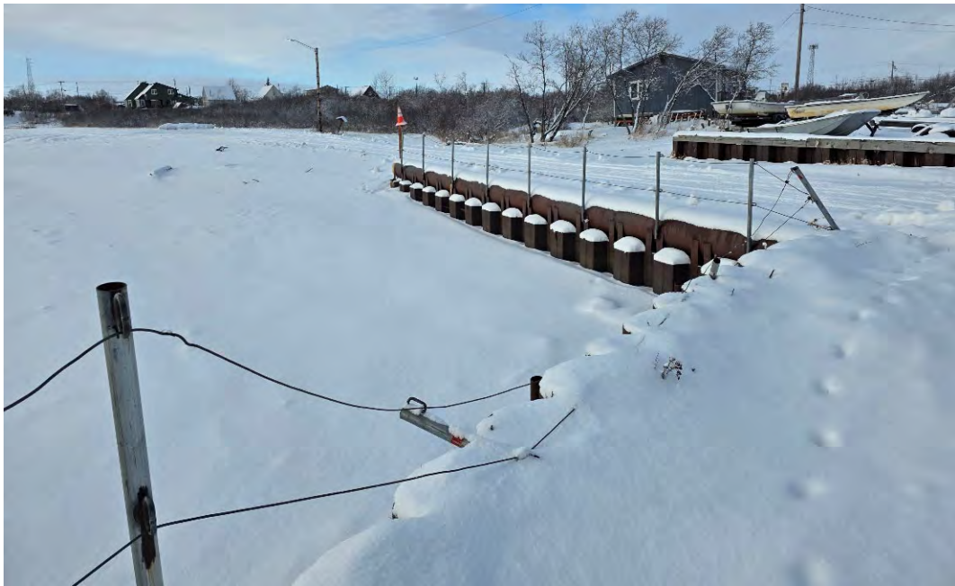
Photo 12: 30" pipe, Z-pile wall cap at DS end of 1st Ave Bulkhead at the US extent of the Float Plane Area. Pipe replaced original timber wall cap, PBL STA 69+00, 3 November 2025
