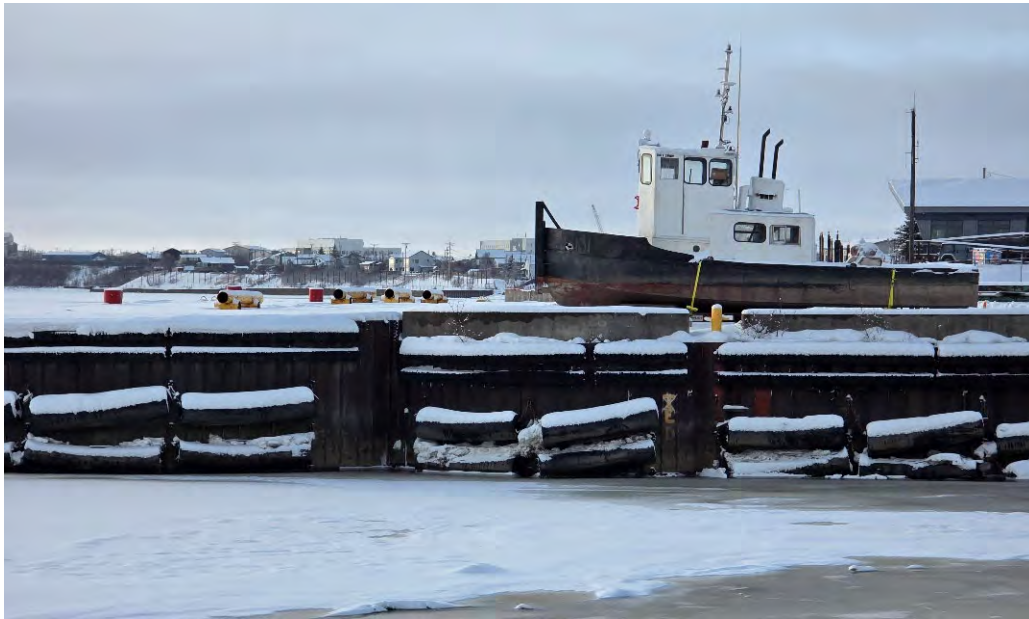
Photo 27: Alternate view of failed area of piles adjacent to City Dock, 3 November 2025, Approx. SCL STA 10+00, 3 November 2025
