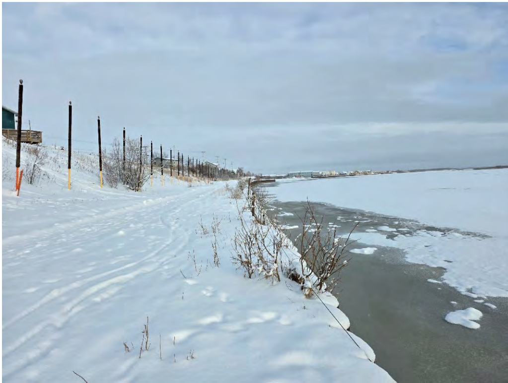
Photo 14: 1st Avenue Bulkhead looking US, failing fence and damaged thermosiphons, with snow covered, PBL STA 73+00, 3 November 2025
