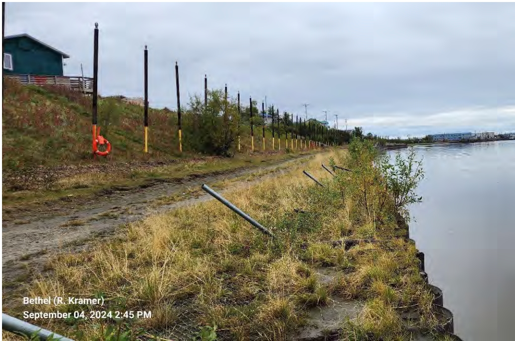
Photo 13: 1st Avenue Bulkhead looking US, failing fence and damaged thermosiphons, PBL STA 73+00
