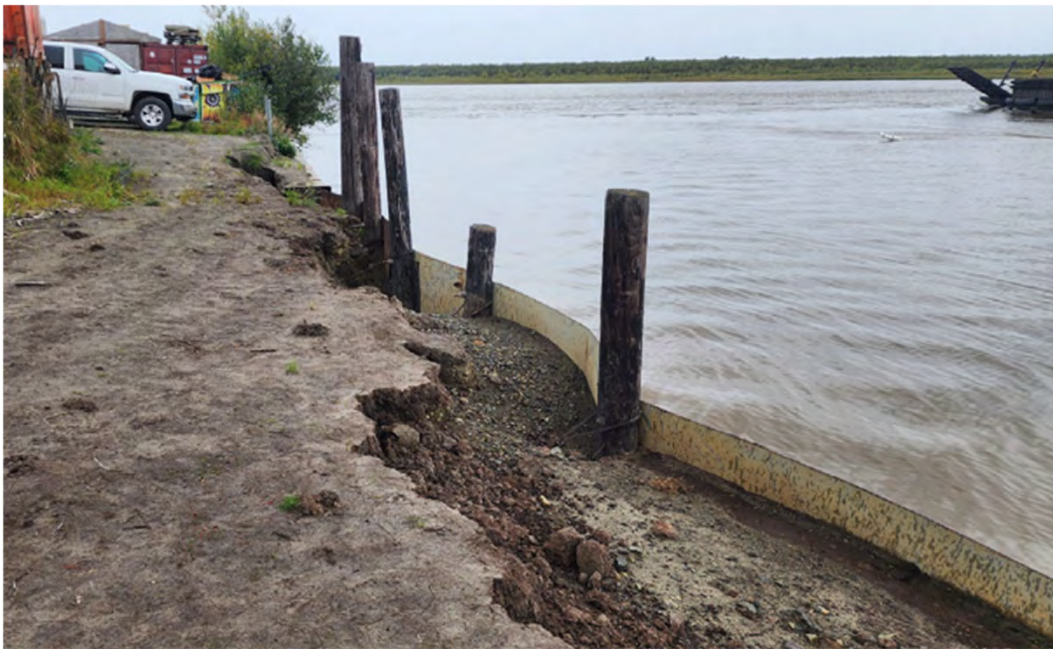
Photo 32: Failing sheet pile on upstream side (relative to the Kuskokwim River) of Brown's Slough, Approx. SCL STA 10+00
