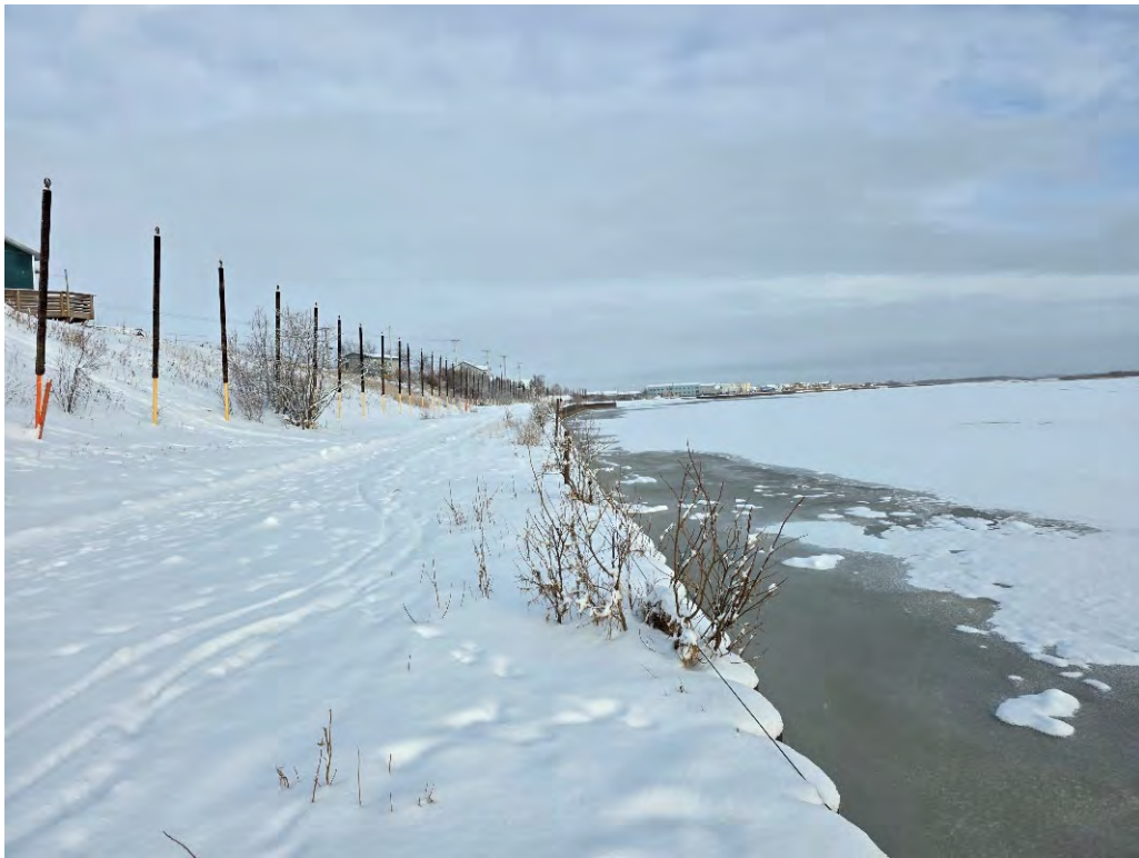
Photo 14: 1st Avenue Bulkhead looking US, failing fence and damaged thermosiphons, with snow covered, PBL STA 73+00, 3 November 2025
