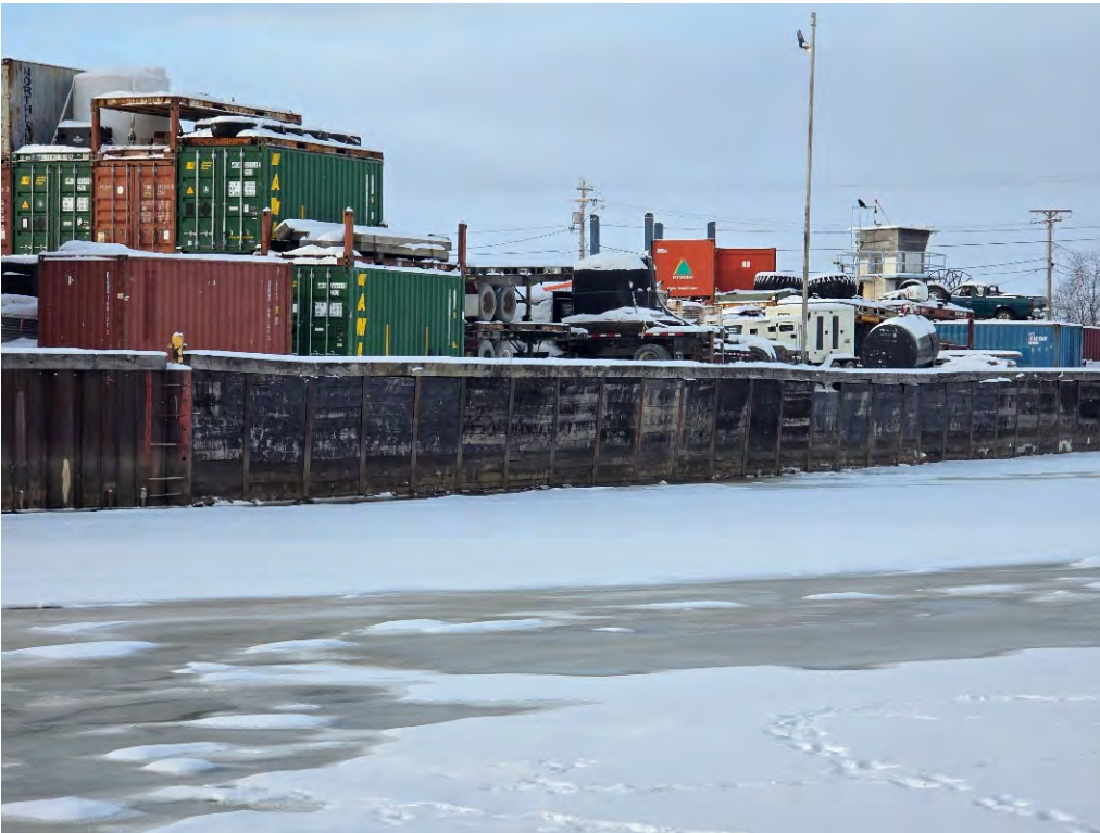
Photo 30: Failing retaining wall on downstream side (relative to the Kuskokwim River) of Brown's Slough, Approx. SCL STA 10+00
