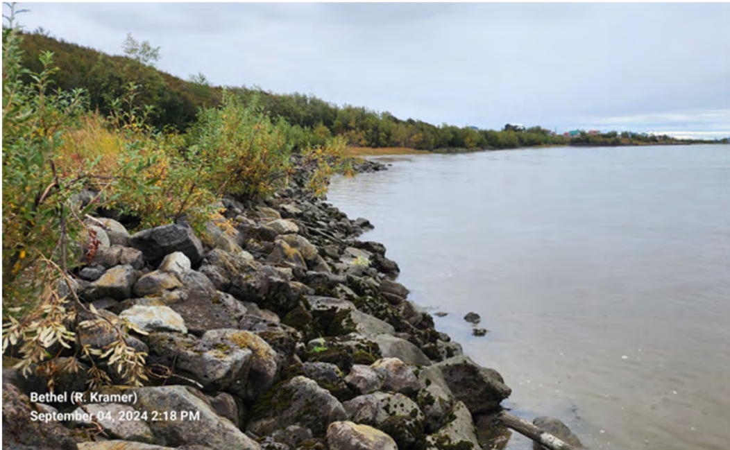
Photo 7: Typical conditions along the rock revetment US from Beach 2 where tree cutting has been completed, Approx. PBL STA 32+00
