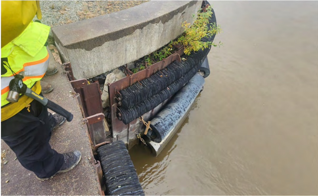
Photo 25: Failed sheet pile interlocks at US end of City Dock, photo taken 4 September 2024 at 1543, Approx. PBL STA 93+40
