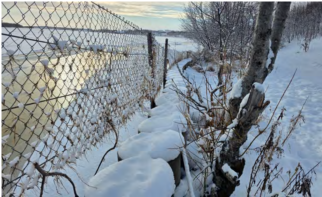
Photo 10: Bowing of 24-in pipe piles downstream, snow-covered, PBL STA 50+00, 3 November 2025
