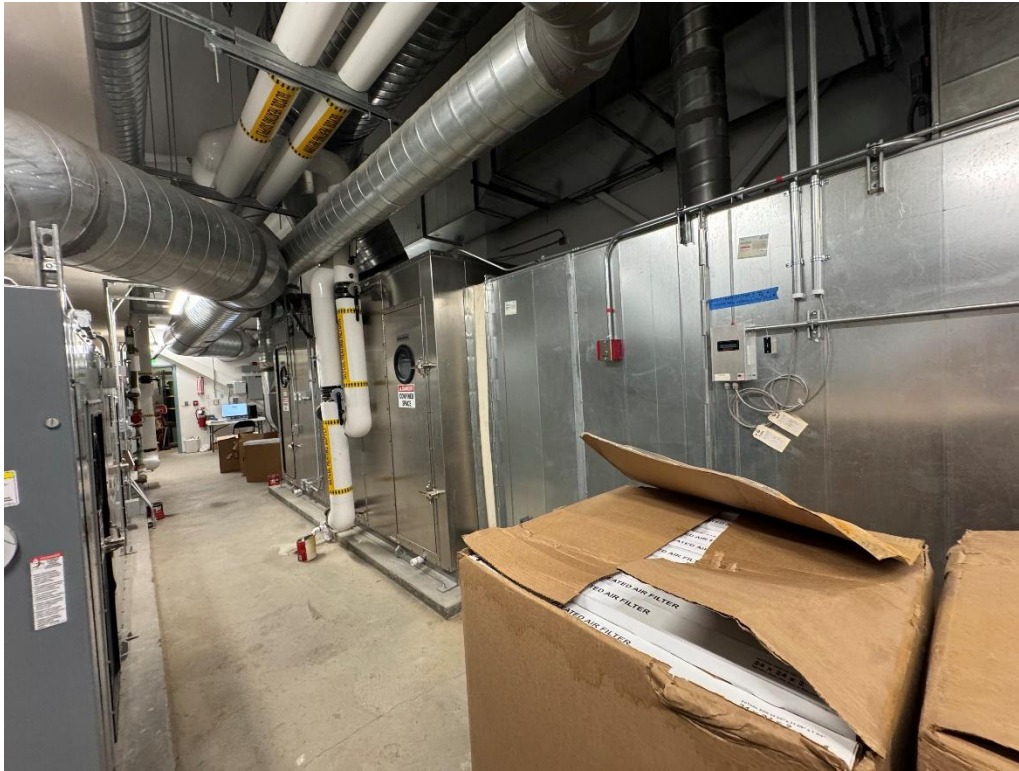
AHUs in the equipment platform
