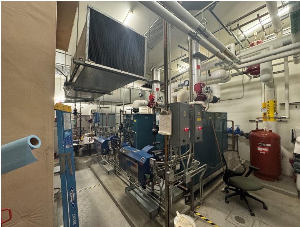
Boiler room, well insulated piping
