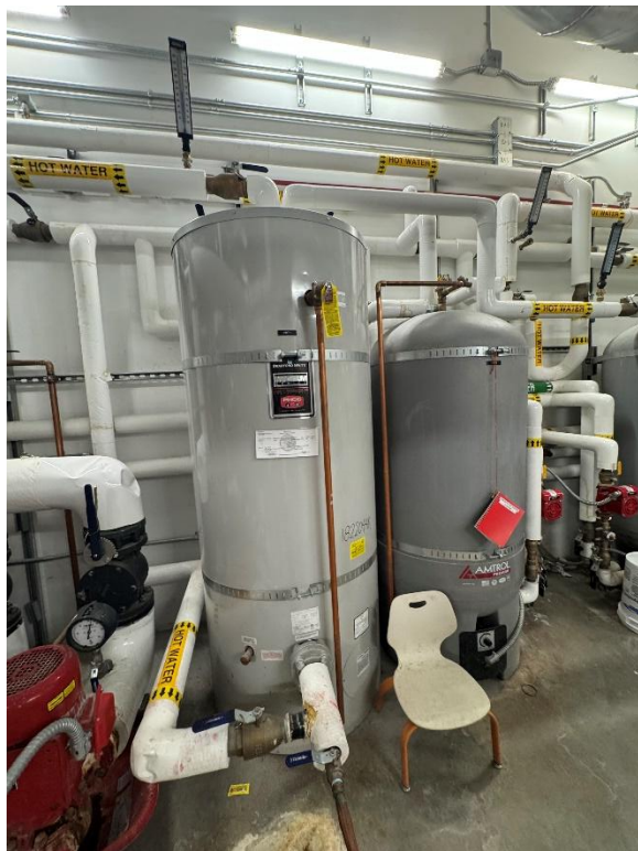
Indirect hot water generator and storage tank
