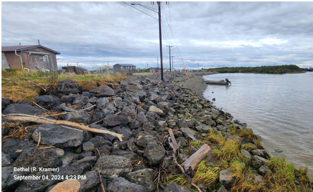
Photo 24: Facing US from US end of East Bulkhead along Small Boat Harbor entrance channel
