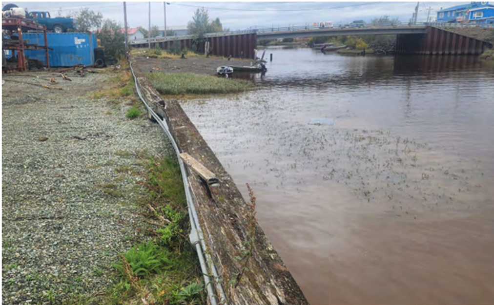
Photo 29: Failing wooden retaining wall and railing failing on downstream side (relative to the Kuskokwim River) of Brown's Slough, Approx. PBL STA 94+00
