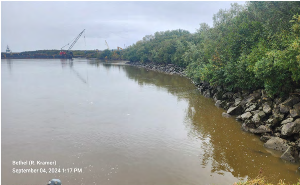
Photo 3: Facing DS from DS end of the Petro Dock near PBL STA 16+50
