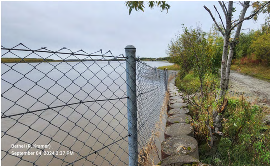
Photo 9: Bowing of 24-in pipe piles downstream, PBL STA 50+00
