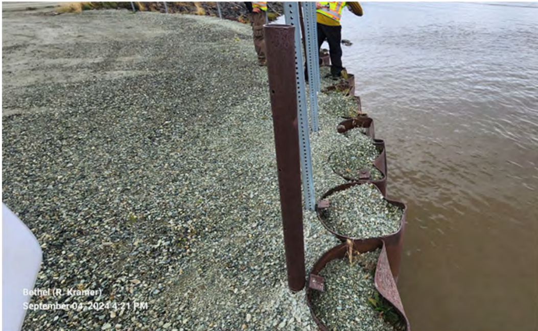
Photo 21: Gravel surfacing appears to have helped block surface drainage path between filter fabric and washout protection angles noted in past reports, Approx. SCL STA 20+50
