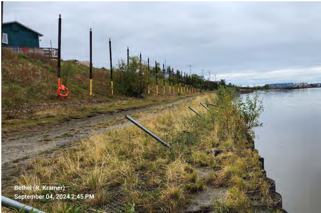
Photo 13: 1st Avenue Bulkhead looking US, failing fence and damaged thermosiphons, PBL STA 73+00
