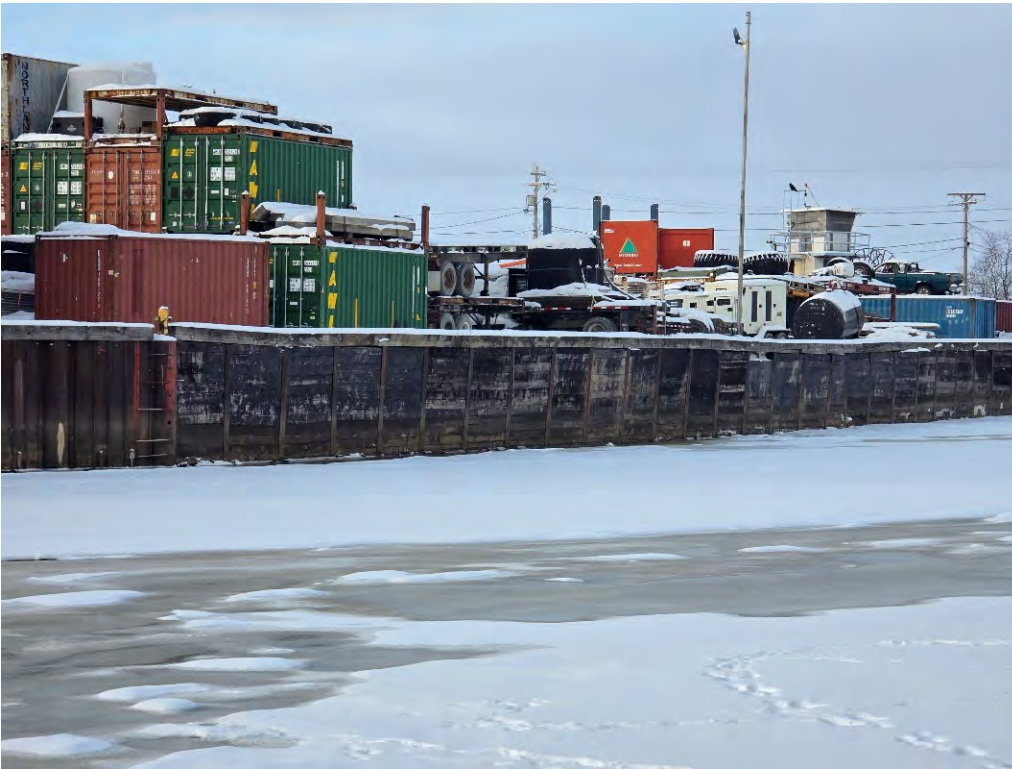
Photo 30: Failing retaining wall on downstream side (relative to the Kuskokwim River) of Brown's Slough, Approx. SCL STA 10+00
