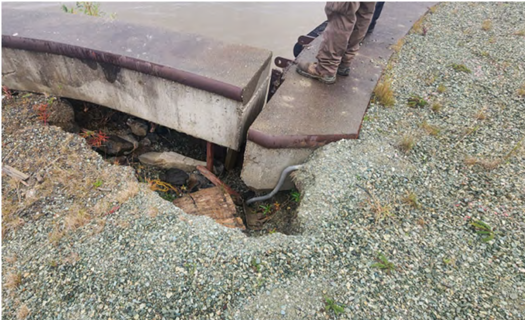
Photo 26: Alternate view of failed area of piles adjacent to City Dock, photo taken 4 September 2024 at 1543, Approx. PBL STA 93+40
