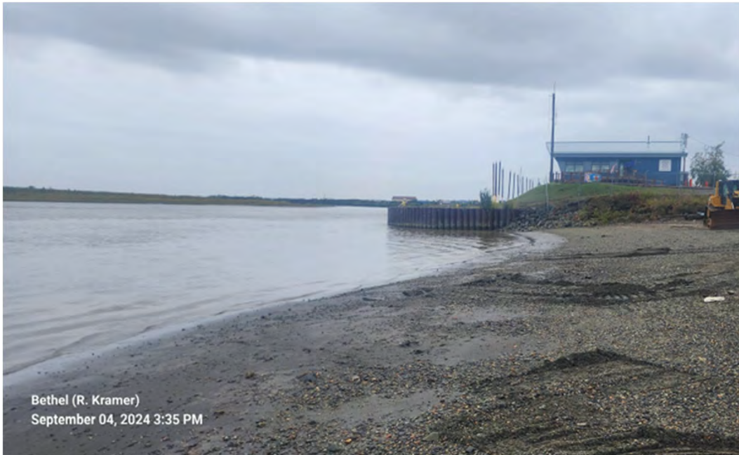
Photo 15: US end of 1st Ave Bulkhead at Beach 1, looking DS at Port Office, all appears stable, PBL STA 90+00
