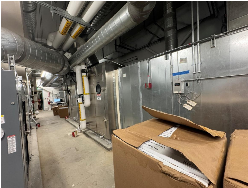
AHUs in the equipment platform
