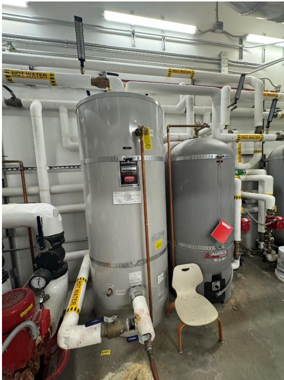
Indirect hot water generator and storage tank
