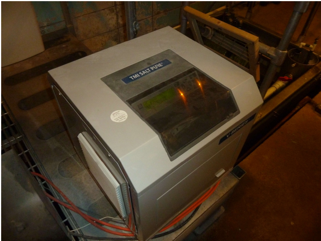
Salt system for water sanitization
