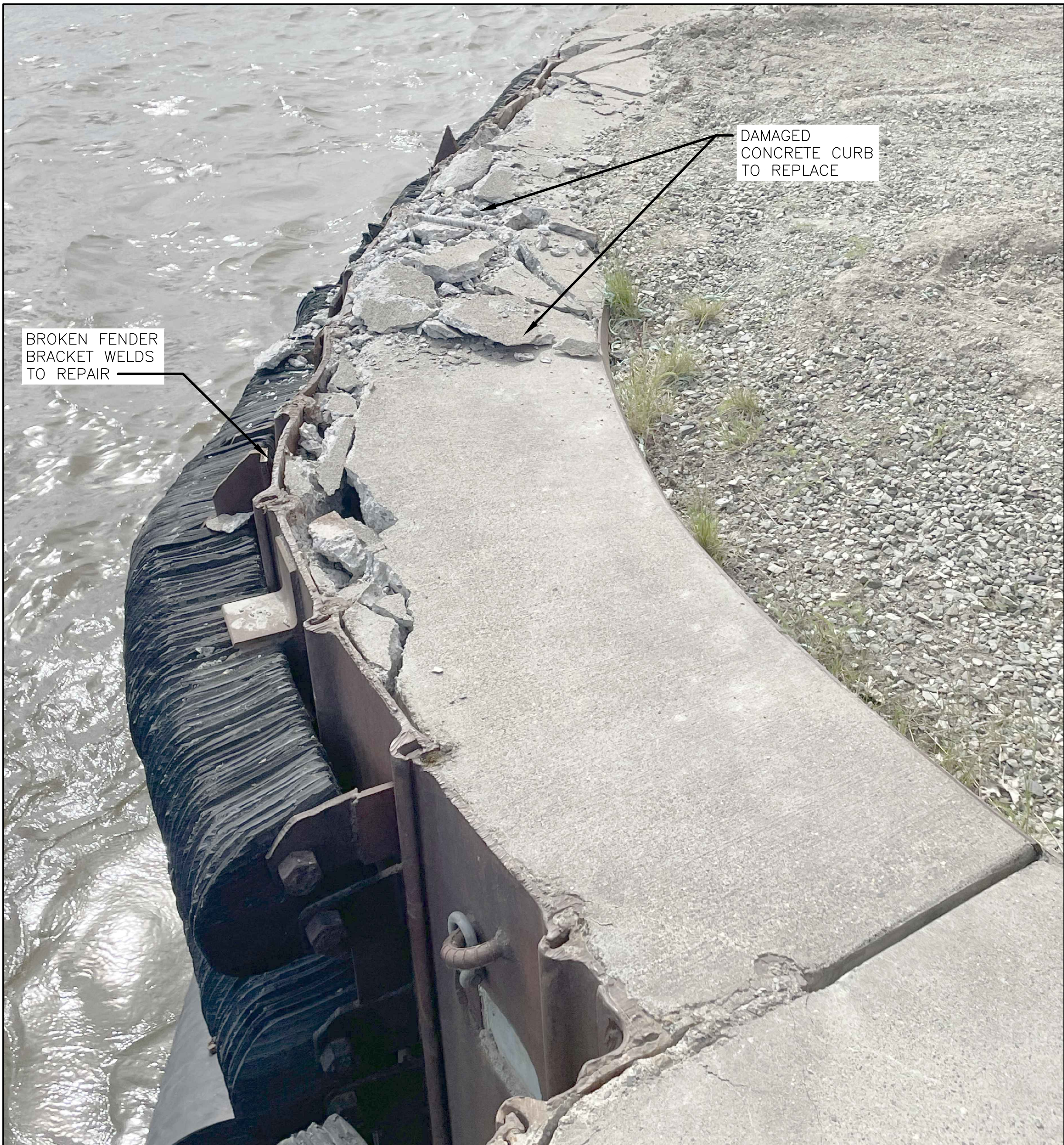
VIEW B-B FIGURE OF DAMAGE NO SCALE
