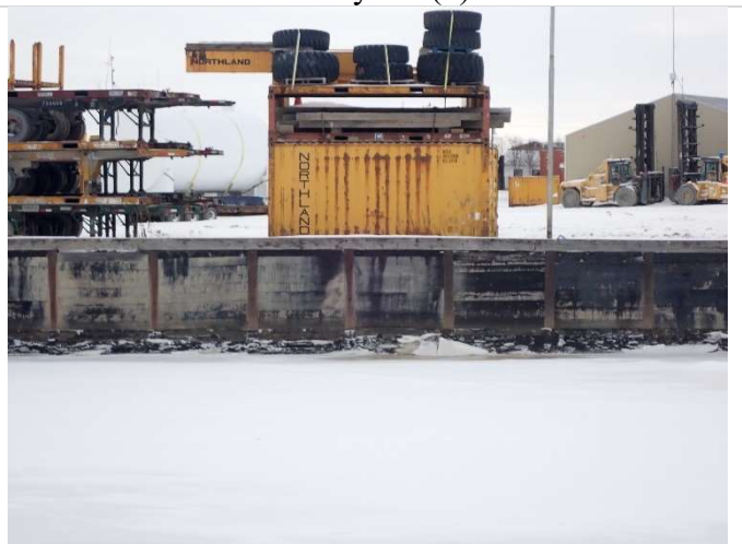
Differential settlement or jacking along timber wall
