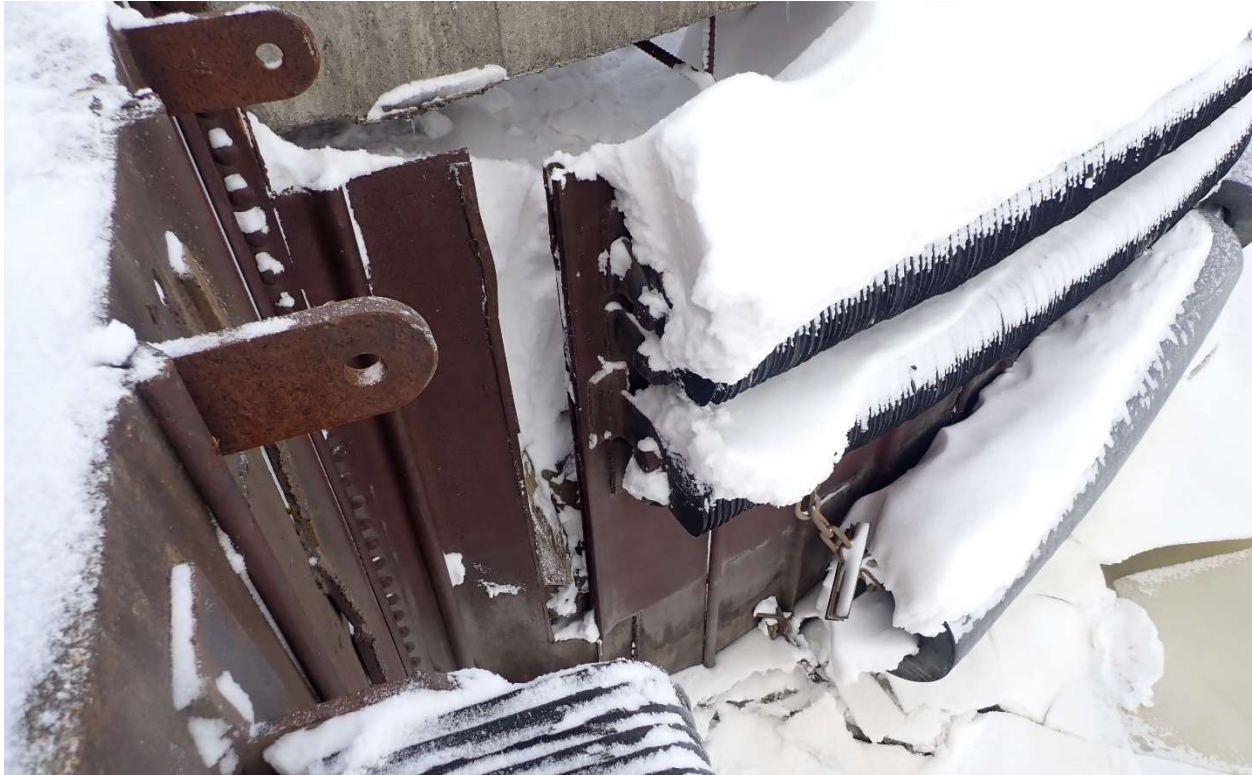
Photo 4: Damaged East Wall Sheet Pile
