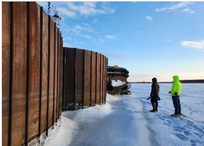
Leaning closure wall between closed cell, CC4, and open cell, OC1. Photo taken in Dec inspection when the ice was thick enough for foot traffic along the east and west walls.
