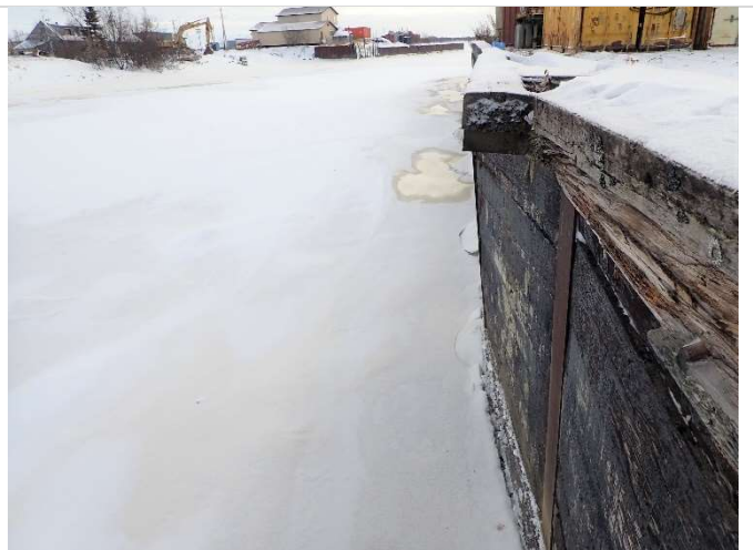
Evidence of failed tie-back along timber wall and damaged timber bullrail
