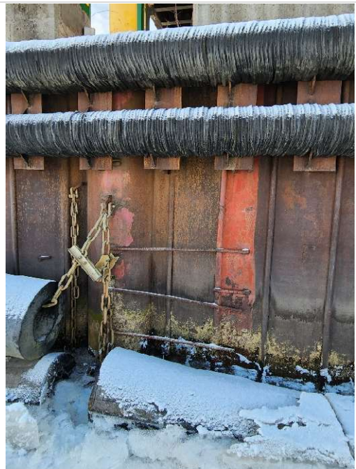
Safety ladder at soldier pile S37
