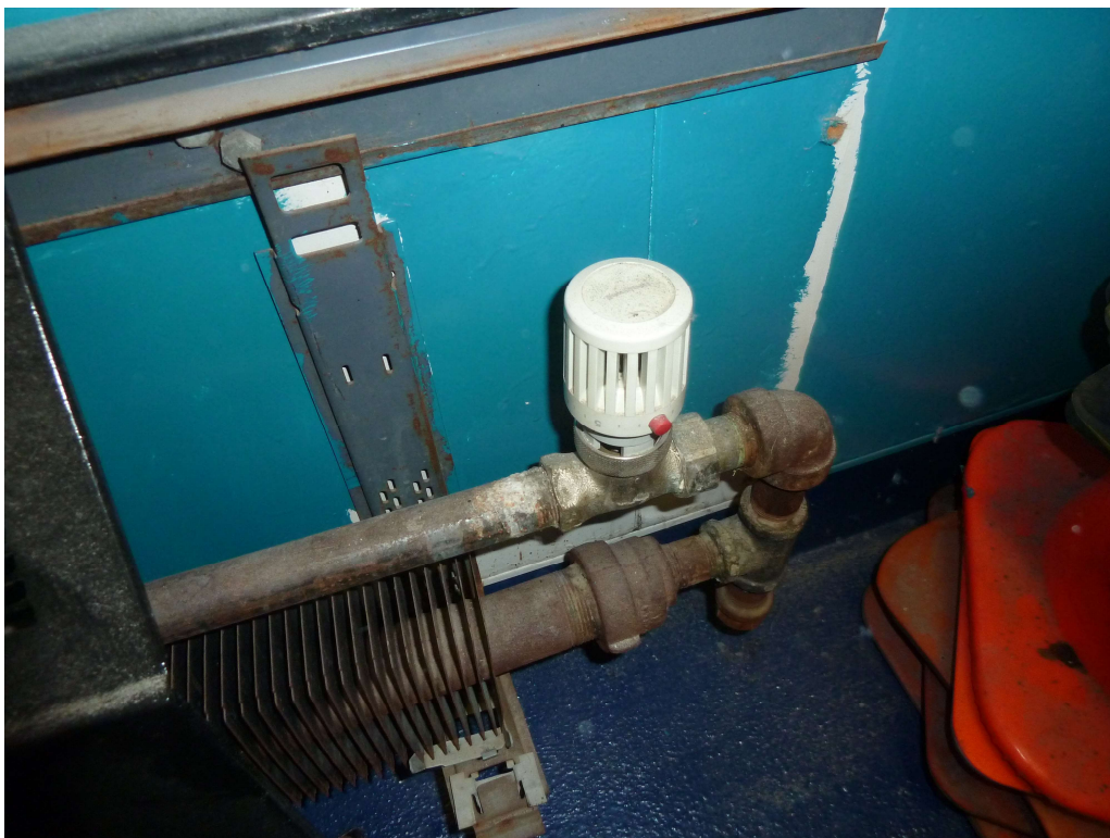
Typical manual thermostatic control valve on fintube baseboard heaters
