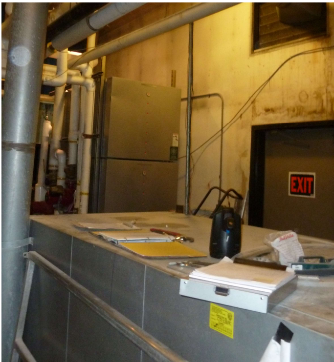
Hot water generators in background, boiler in foreground
