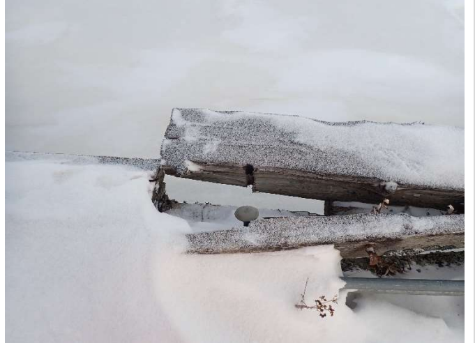
Damaged timber bullrail along timber wall
