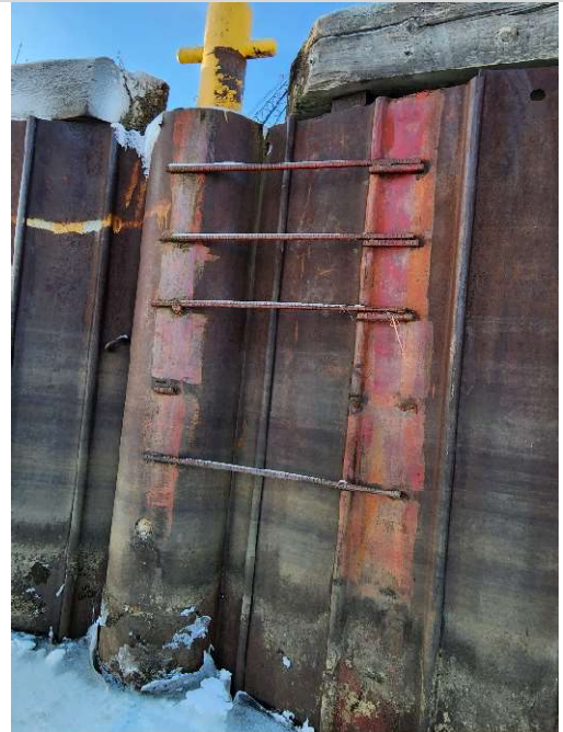
Safety ladder at soldier pile S19
