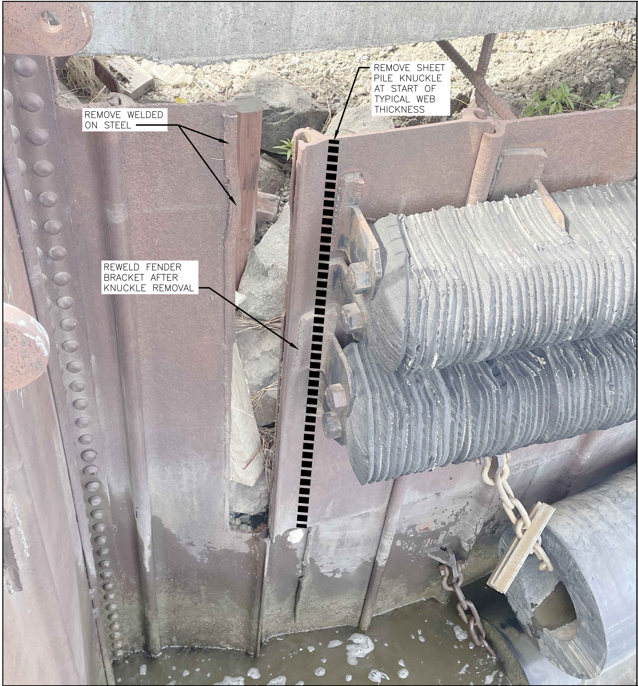
VIEW A-A FIGURE OF DAMAGE NO SCALE
