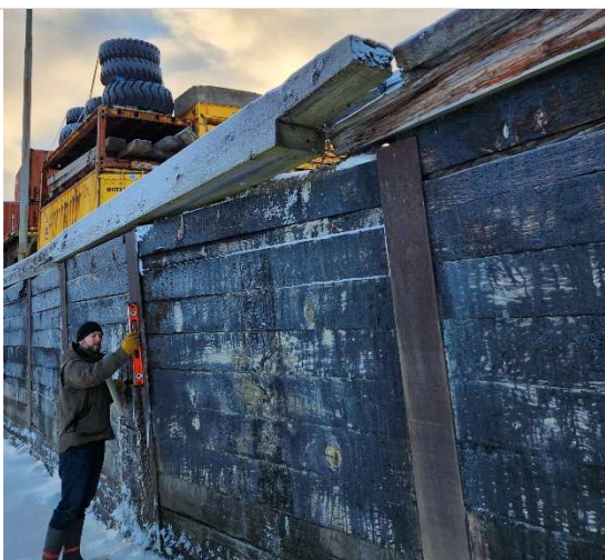
Evidence of failed tie-back along timber wall at soldier pile T17
