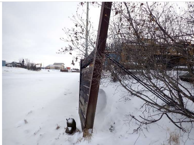
HP leaning shoreward as the pile frost jacks while still restrained by the (2) tie-backs
