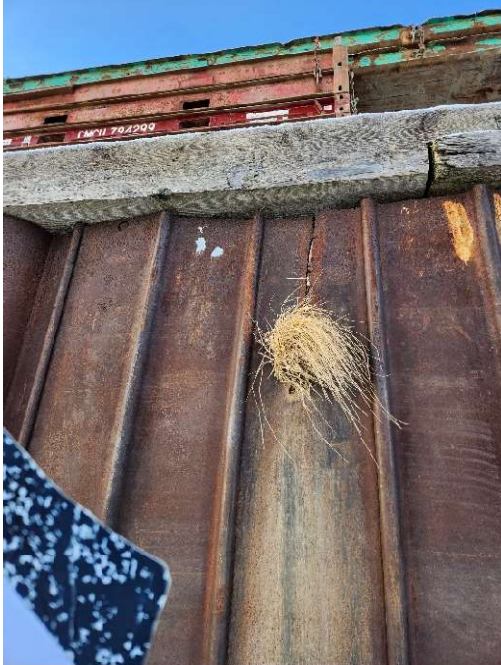
Damaged sheet pile near soldier pile S11
