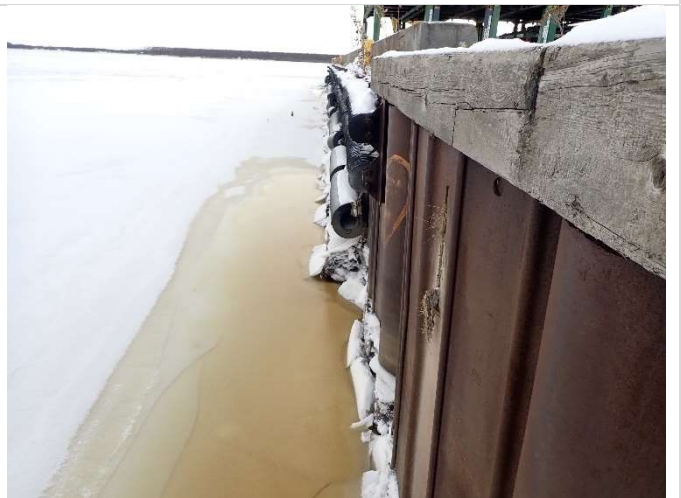
Damaged sheet pile on east wall
