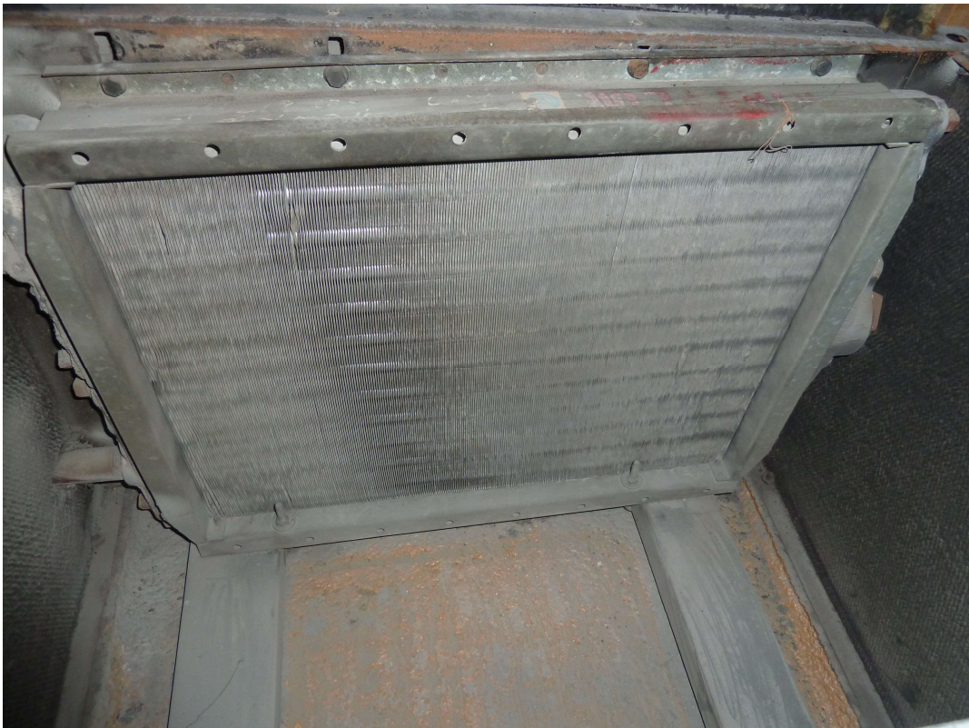
AHU-2 heating coil should be cleaned inside and out
