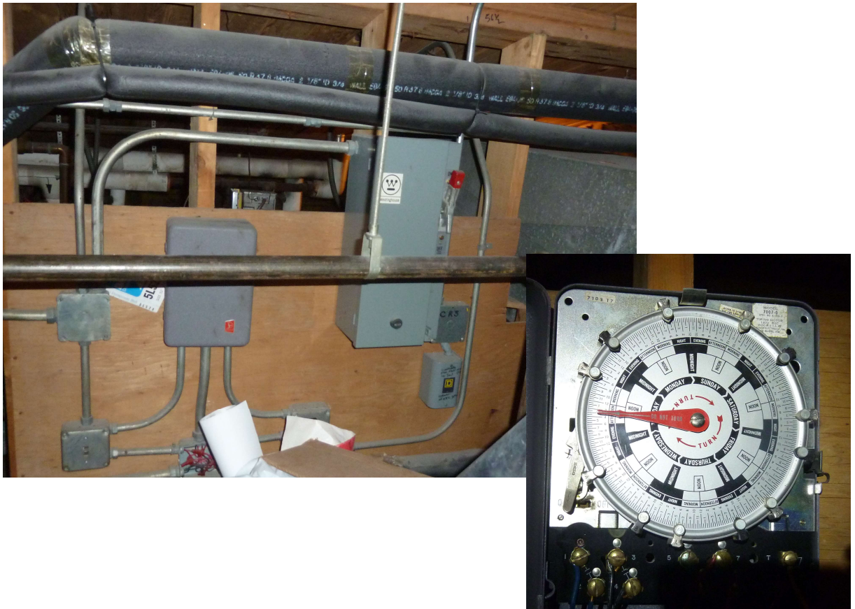
Control panel for AHU-2 above; time clock for AHU-2 (right) is not in use
