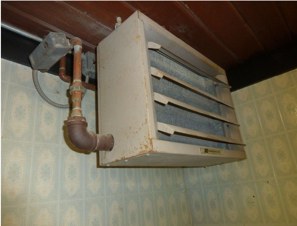
Unit heater typical of Men's and Women's locker rooms. Note wall switch is turned off due to occupancy complaints of noise and air blowing on wet bathers
