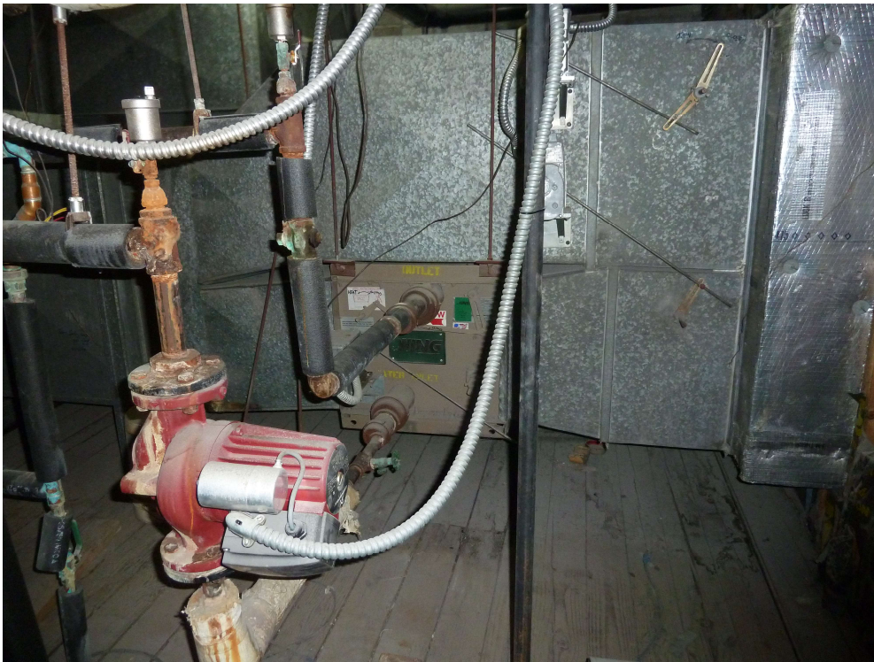
AHU-1 primary heating coil
