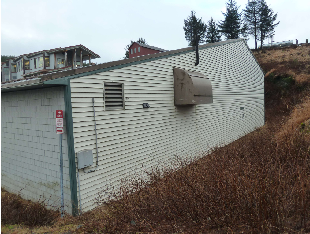
AHU-1 inlet in center, exhaust vent at left; exhaust has been unused since the fan was de-commissioned
