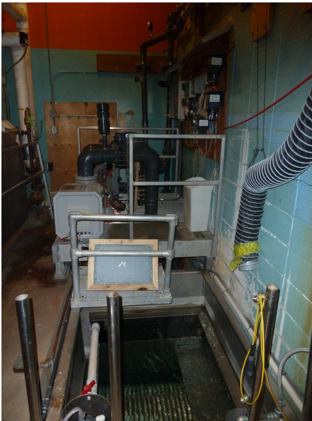
Filter pit and water temperature controller
