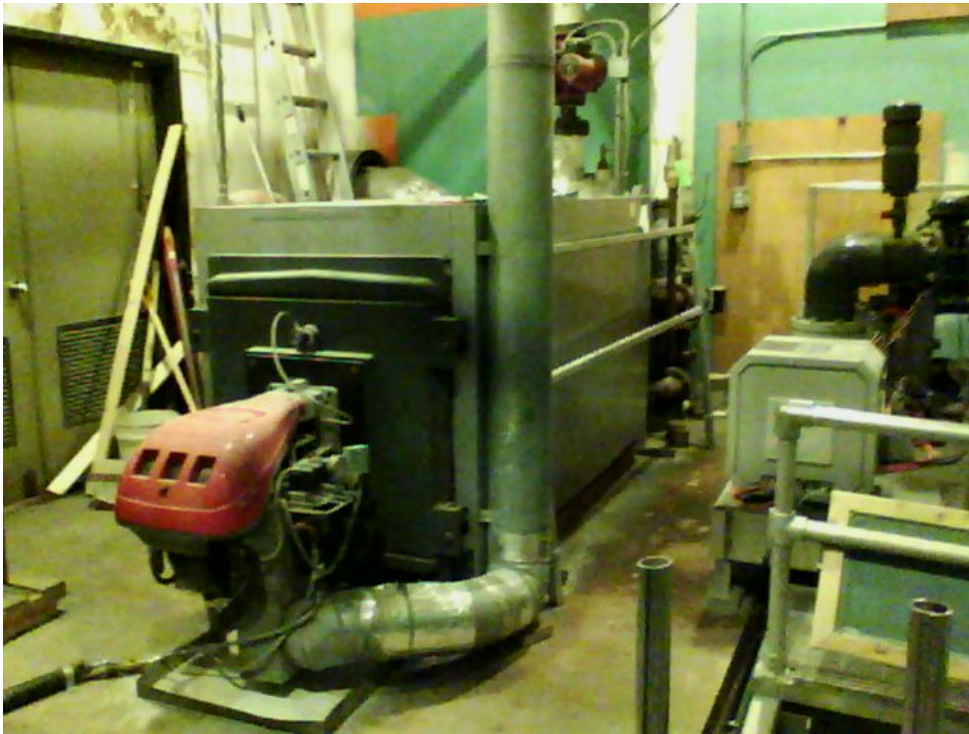
Boiler appears to be in good condition
