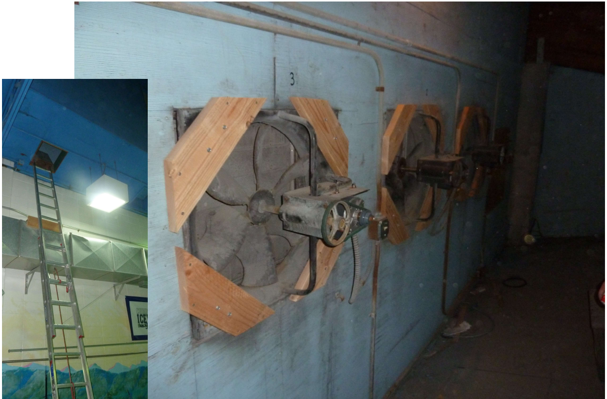
Clearstory exhaust fans; #3 is manually turned off, #2 and #1 seem to run continually
