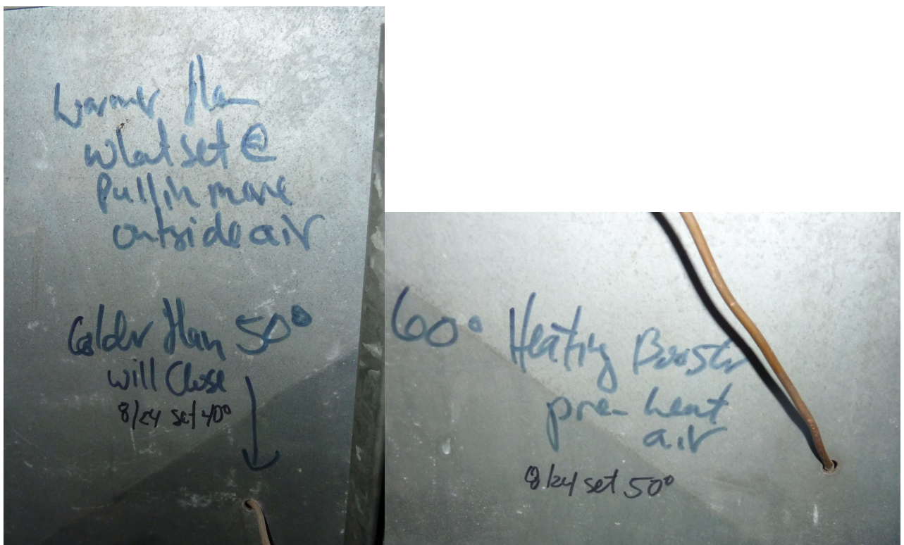
Pre-heat and main heating set points have been altered
