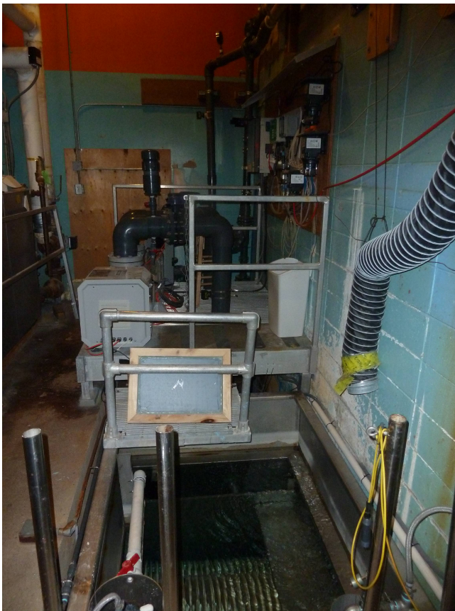
Filter pit and water temperature controller
