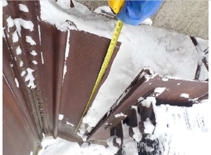
Length of damaged sheet pile section
