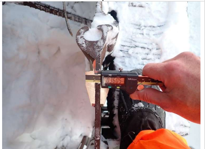
East wing wall PS28 web thickness remaining at top of wall
