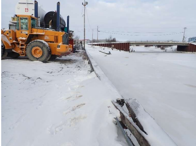
Damaged timber bullrail along timber wall
