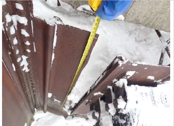
Length of damaged sheet pile section
