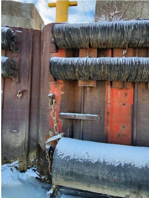
Safety ladder at soldier pile S46
