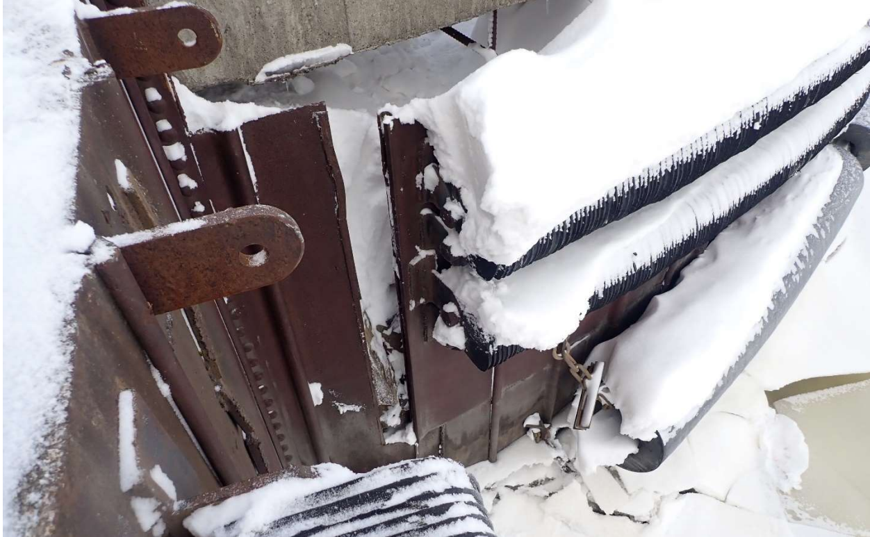
Photo 4: Damaged East Wall Sheet Pile
