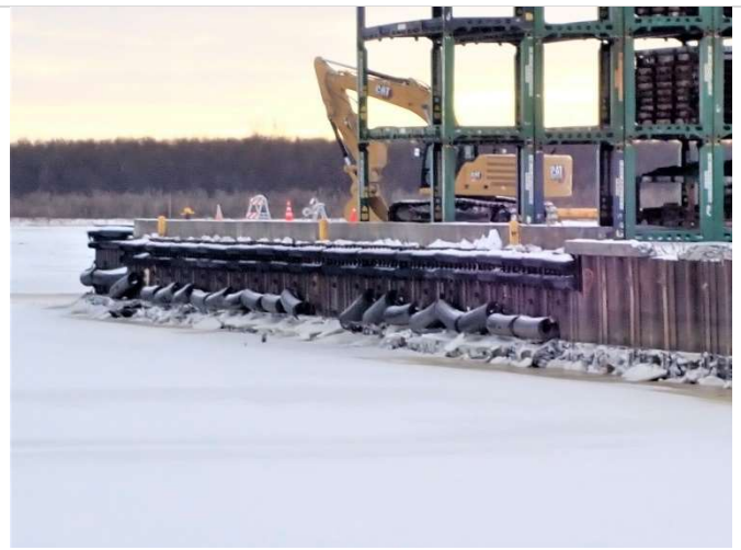
Fendering on east sheet pile wall
