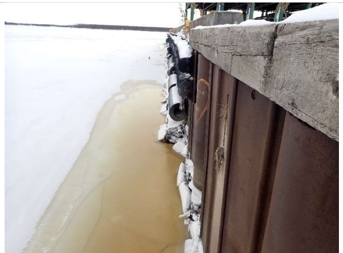
Damaged sheet pile on east wall
