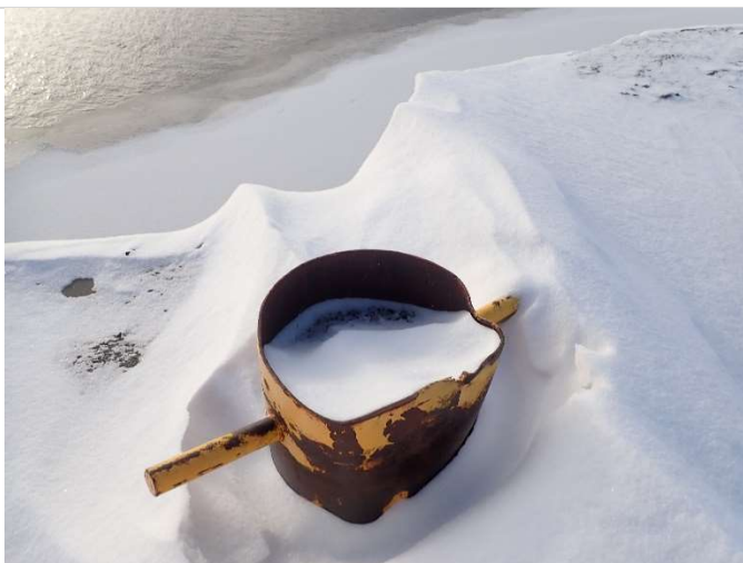
Damaged 24" dia pipe pile bollard at closed cell #2
