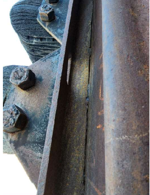
Crack indication at connection between fendering bracket and wall near start of east wall fendering
