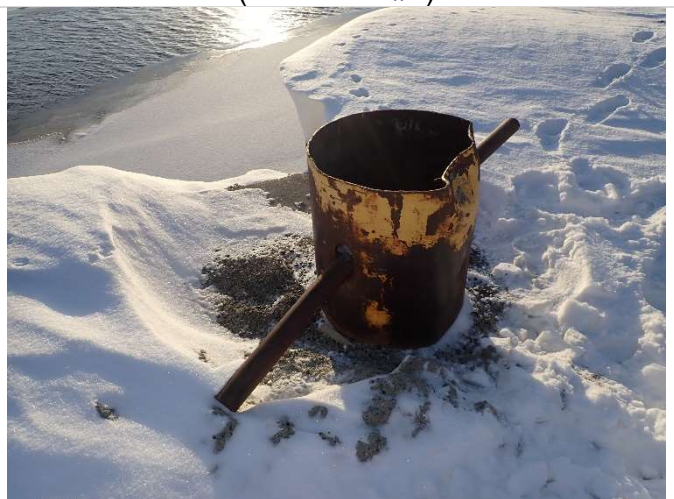
Damaged 24" dia pipe pile bollard at closed cell #3. Hole has been drilled through pile-pile with a 3" dia bar inserted through the pile
