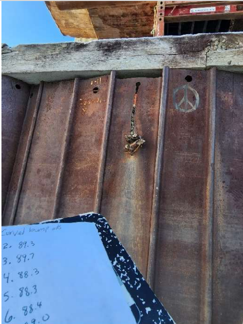
Damaged sheet pile near soldier pile S13
