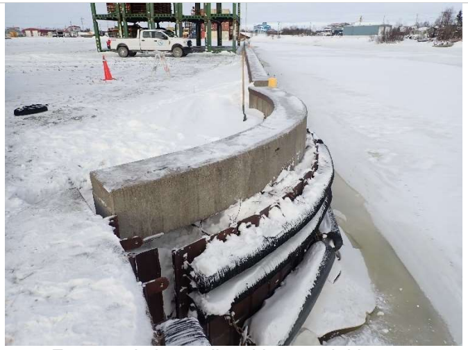
Fractured sheet pile with material loss at connection between east wing wall and dock closed sheet pile dock cell
