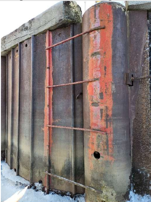
Damaged safety ladder at soldier pile T35 & S1
