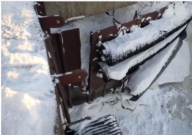
Fractured sheet pile with material loss at east wing wall
