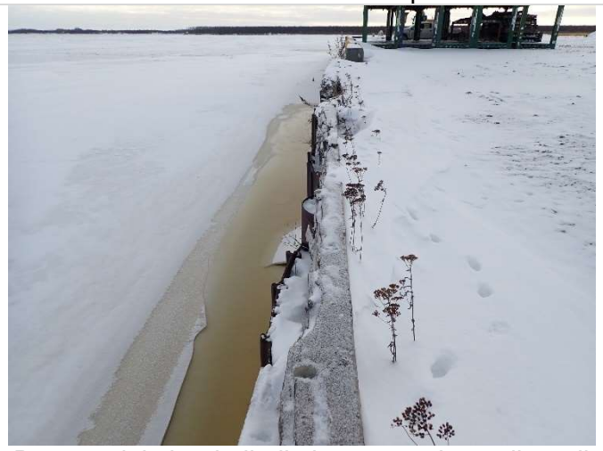
Damaged timber bullrail along east sheet pile wall
