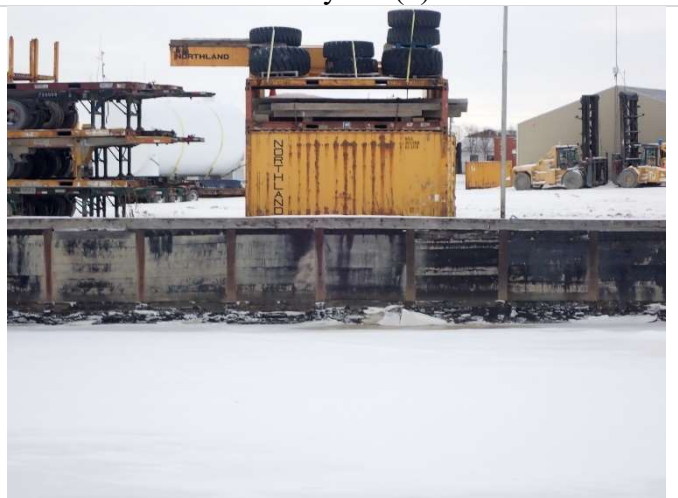
Differential settlement or jacking along timber wall
