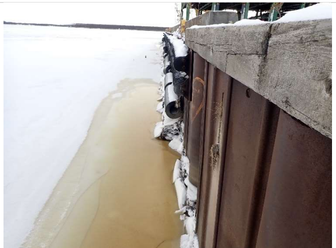
Damaged sheet pile on east wall
