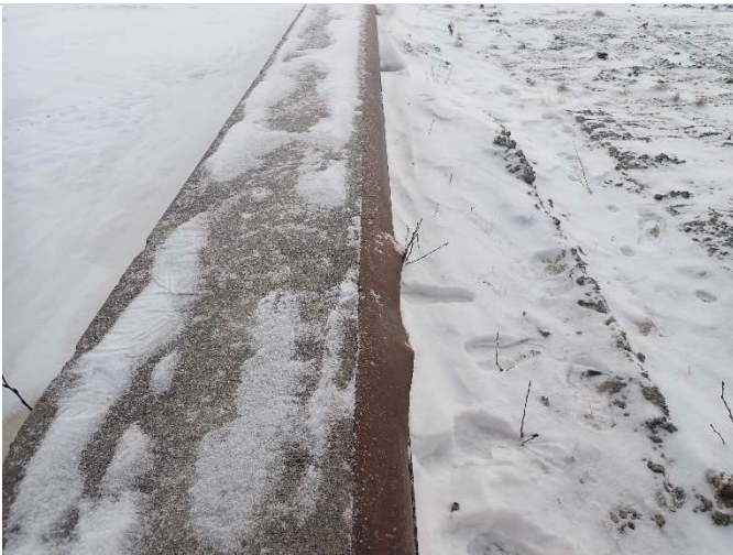
Minor damage to concrete curb metal strip along east wall.
