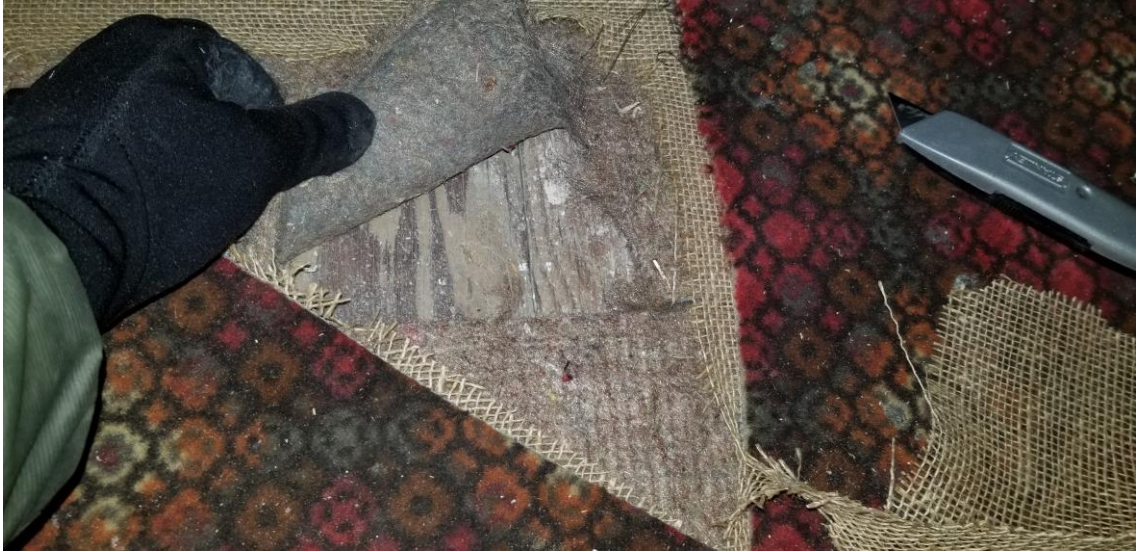
Photo 5: This photo shows the flooring within the building. The carpet was removed in multiple areas and in all instances only bare plywood was beneath.
