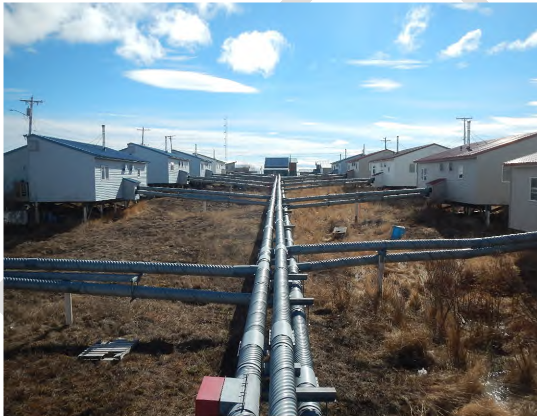
Water and sewer pipes serving homes in the Bethel Heights neighborhood.
