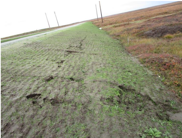
Thaw settlement embankment slope failure from STA 7+00 to STA 7+50, RT (Madilyn's Way).
