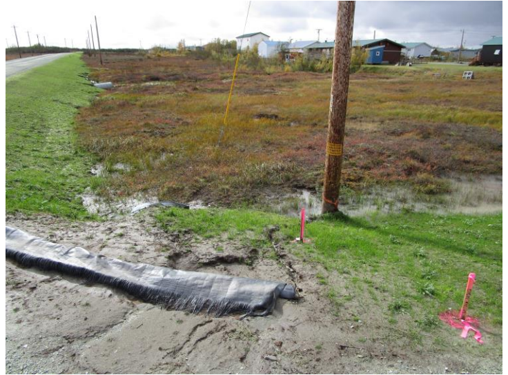
Non-stabilized area along Karis Street near STA 0+40, LT.
