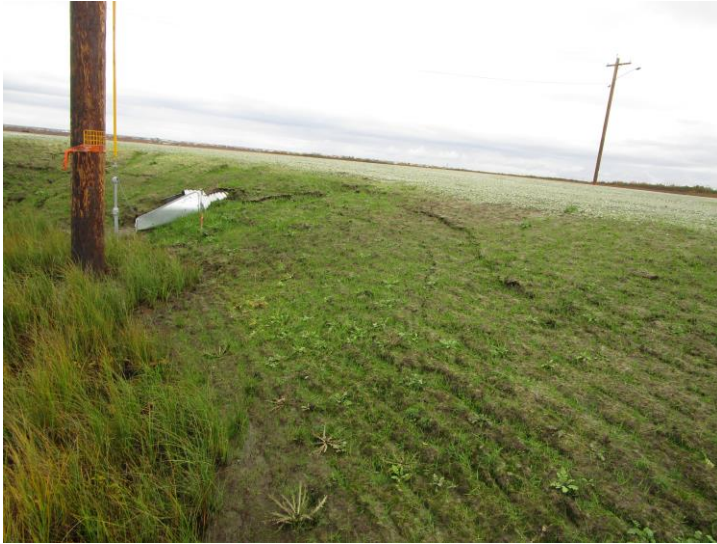
Slumping / thaw settlement embankment slope failure from STA 0+25 to STA 0+75, RT (Karis Street).
