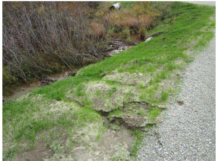
Minor gulleys along Elizabeth Street at STA 0+50, RT.
