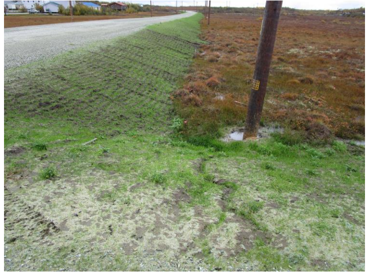
Minor gulleys along Karis Street at STA 16+80, LT.
