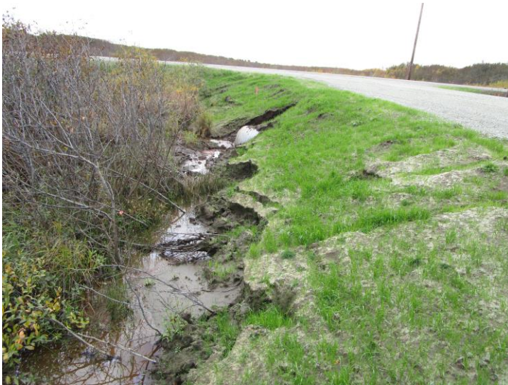
Embankment failure and hydraulic erosion at toe along Elizabeth Street near beginning of project (BOP).
