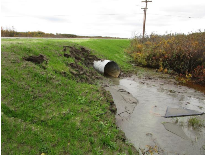
Significant embankment slope failure adjacent to 36-inch CMP culvert pipe outlet near STA 0+75 (Elizabeth Street).
