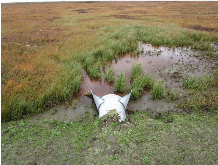
Approx. 3-ft section of 24-inch CMP culvert pipe not backfilled between existing embankment toe and culvert end section (STA 11+90, RT – Karis Street).
