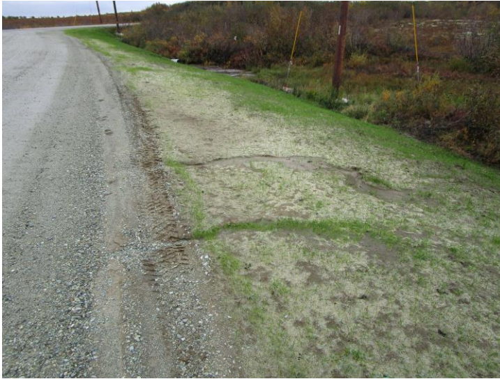
Non-stabilized area along Elizabeth Street near STA 1+50, LT.
