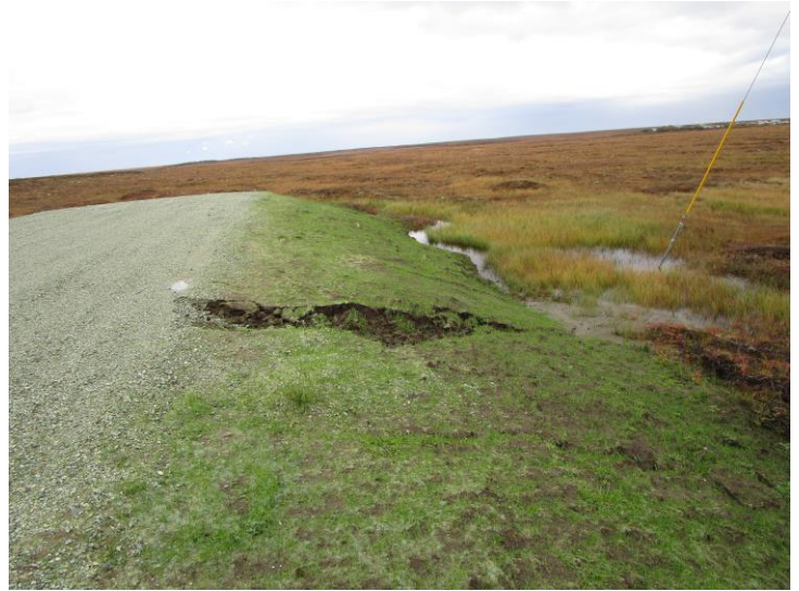
Embankment slope failure along Madilyn's Way at STA 12+50, RT.
