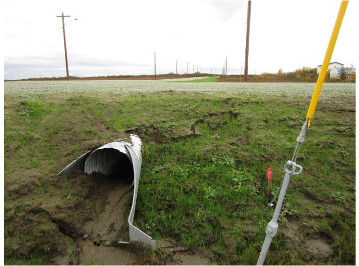
Thaw settlement embankment slope failure at culvert pipe outlet (STA 0+35, RT – Karis Street).
