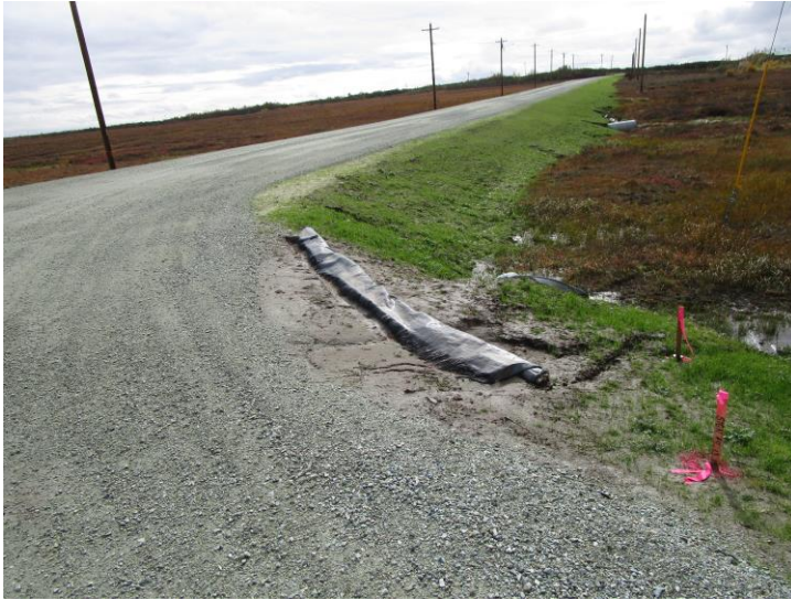
Minor gulleys along Karis Street at STA 0+30, LT.
