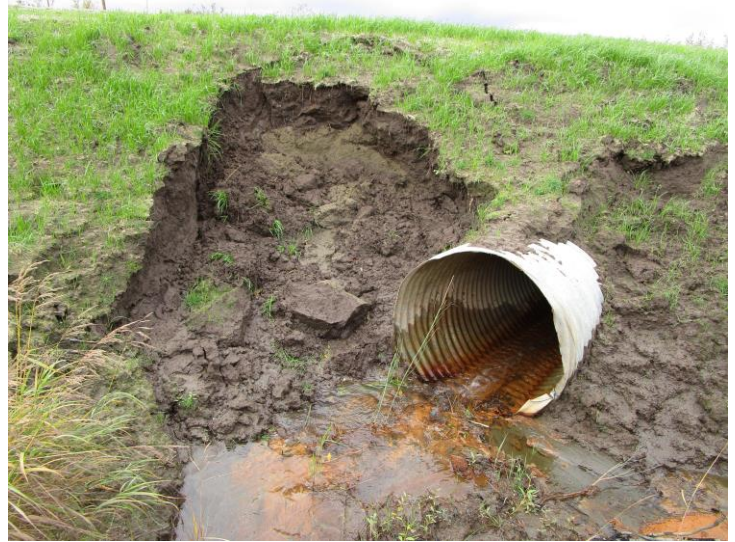
Significant embankment slope failure adjacent to 36-inch CMP culvert pipe inlet near STA 0+40 (Elizabeth Street).
