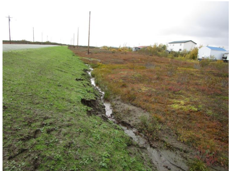
Embankment failure and hydraulic erosion at toe along Madilyn's Way near STA 10+00, LT.
