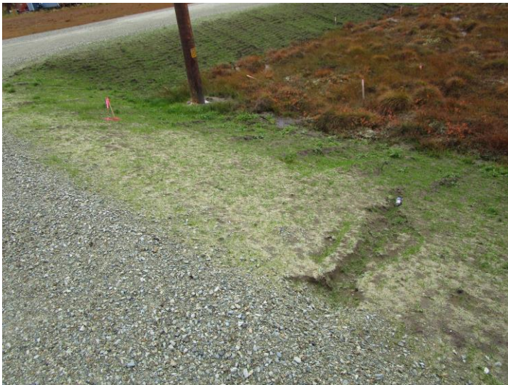
Minor gulleys along Karis Street at STA 17+00, LT.
