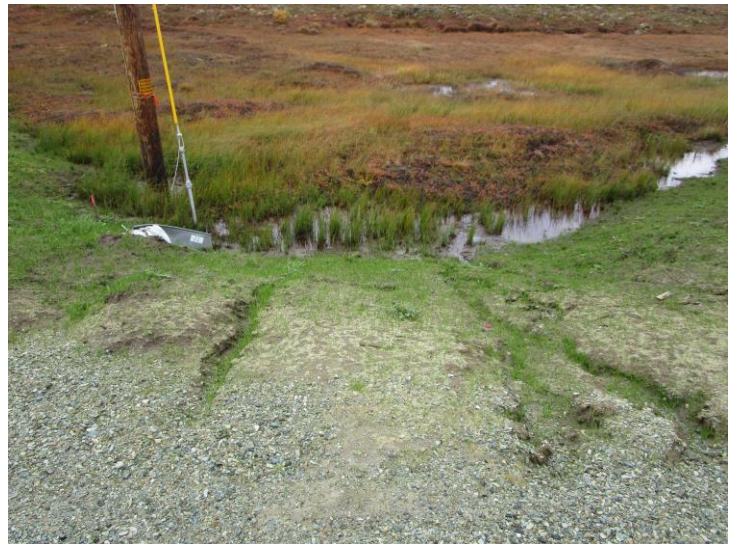
Minor gulleys along Karis Street at STA 0+30, RT.
