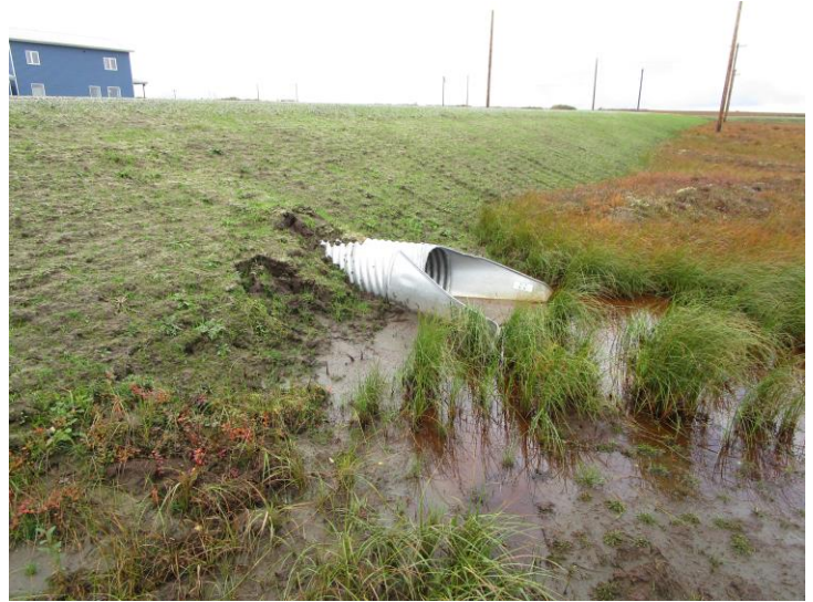
Minor embankment slope failure adjacent to 24-inch CMP culvert pipe outlet at STA 11+90, RT (Karis Street).
