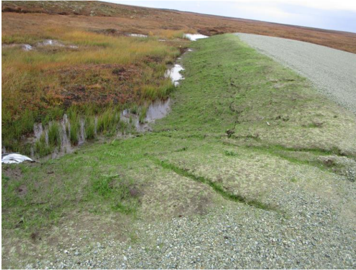
Slumping / thaw settlement embankment slope failure near STA 12+30, LT (Madilyn's Way).
