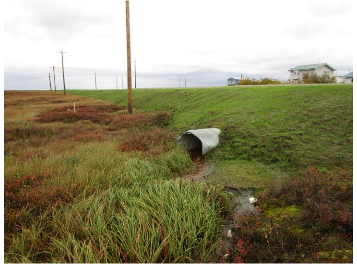
Damaged 36-inch CMP roadway cross culvert at STA 4+92, LT (Elizabeth Street).
