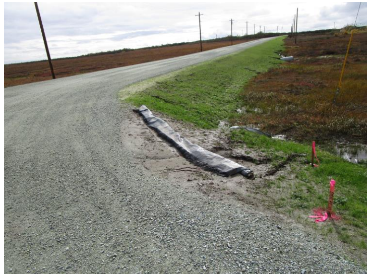
Construction material needing removal at STA 0+30, LT (Karis Street).
