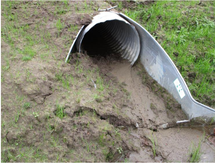
Obstructed 24-inch CMP culvert pipe outlet at STA 0+35 (Karis Street).
