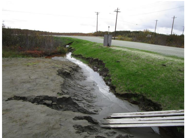
Embankment failure and hydraulic erosion at toe along Elizabeth Street near BOP.
