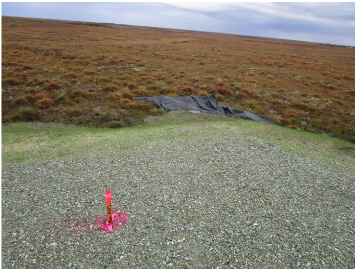
Excess geotextile fabric extending beyond toe of slope at STA 12+40, RT (Elizabeth Street).
